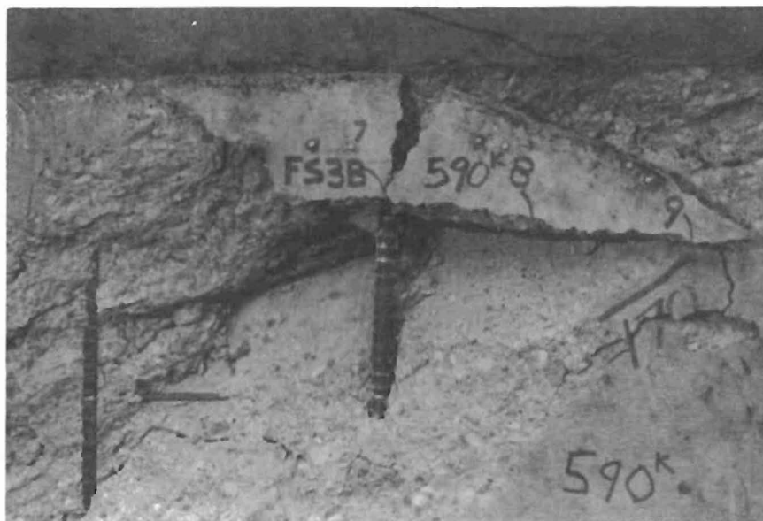
(b) Close up of failure zone. Vertical bar in center has been forced outward
