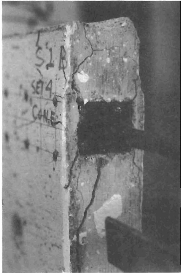
(c) t = 3 in., e = 0.6a (6 in.) after failure. Diagonal cracks propagate from four corners of anchor. Anchorage is forced into web, nonexplosive failure
