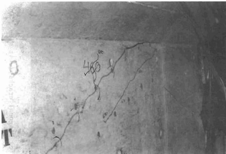
(f) Longitudinal cracks near point of maximum curvature (west side)
