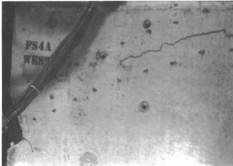
(a) First cracking at point of maximum curvature
