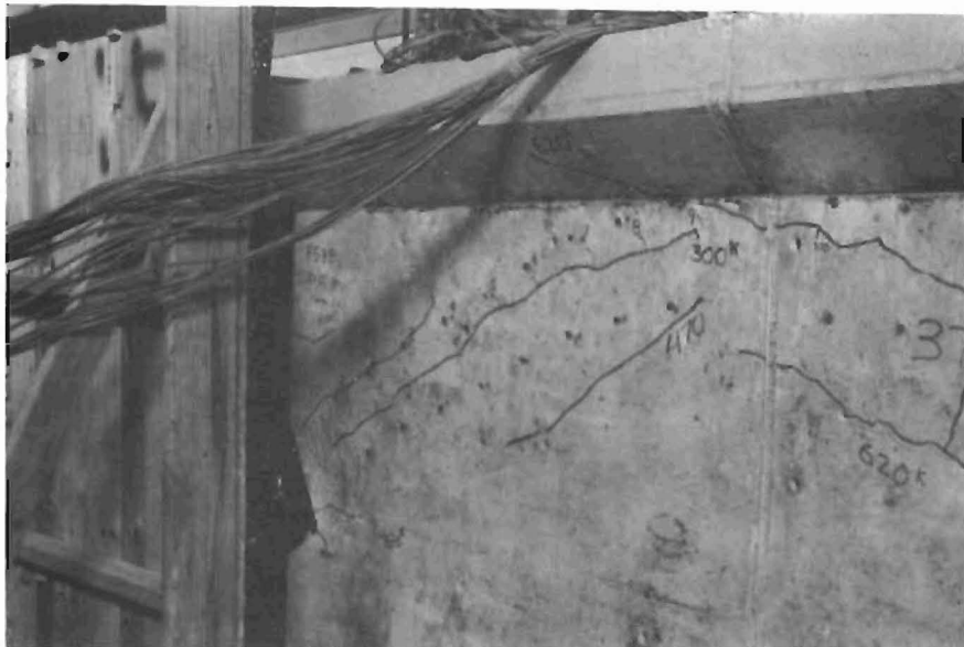
(b) Lower longitudinal crack forms at point of maximum curvature. Upper and lower diagonal cracks form shortly thereafter
