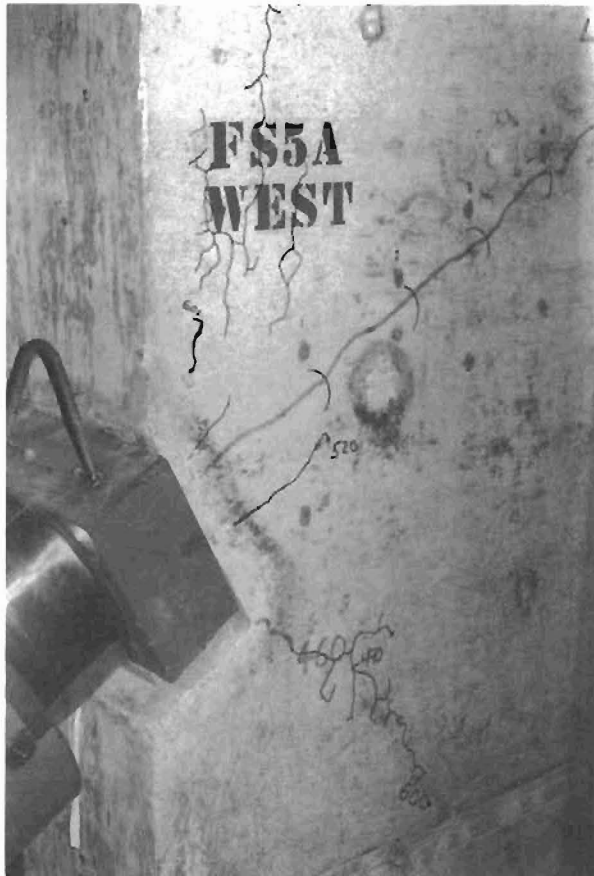
(c) Diagonal cracks, west side
