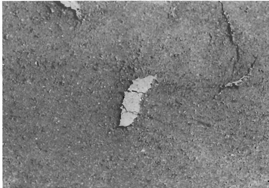
Figure 29 Spalling of Blended Recycled Surface
