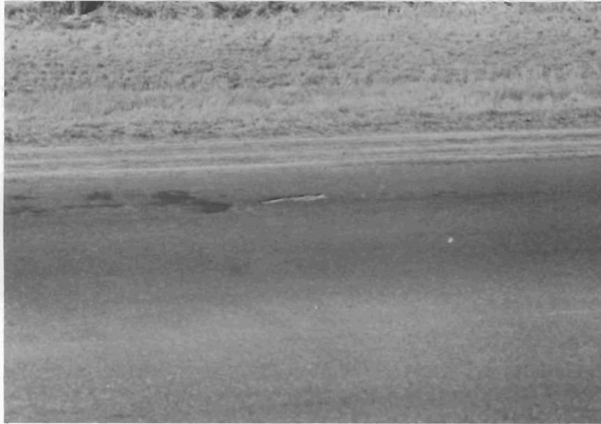
Figure 20 Spalled Pavement Surface
