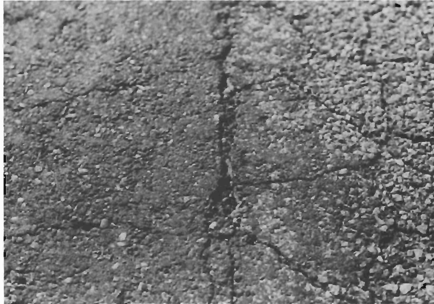
Figure 27 Longitudinal Edge Crack Between Recycled Surface and Shoulder
