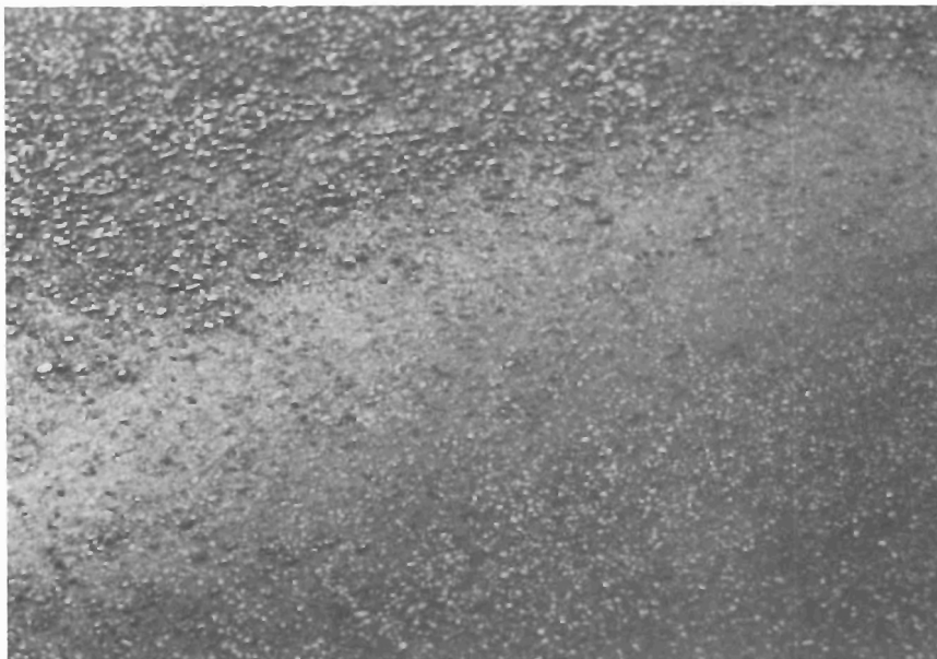
Figure 3 Comparison of Wheel Path Texture with that of Remaining Roadway
