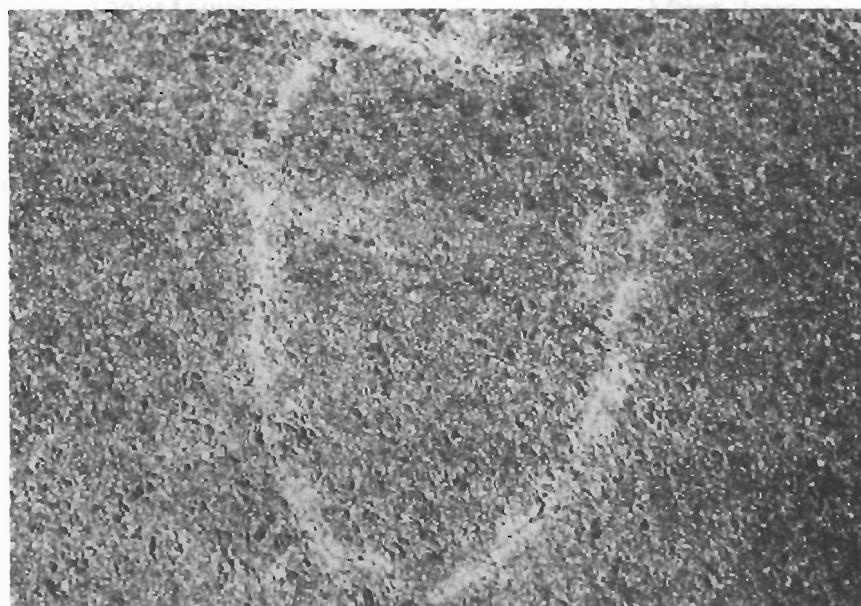
Figure 19 Fines Pumped to Surface of Roadway
