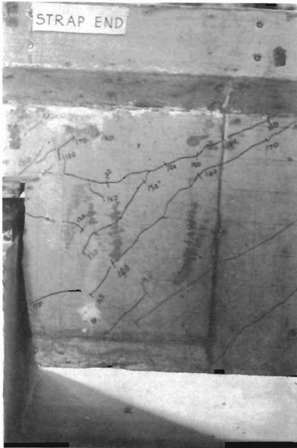
(a). Cracks at strap end.
