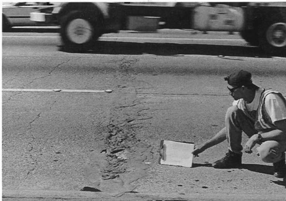
Figure 2.16 Example of a failed joint on IH-10
