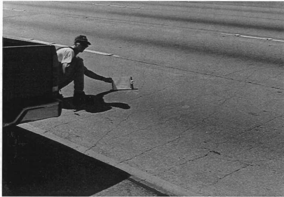
Figure 2.12 Typical cracking of eastbound lanes
