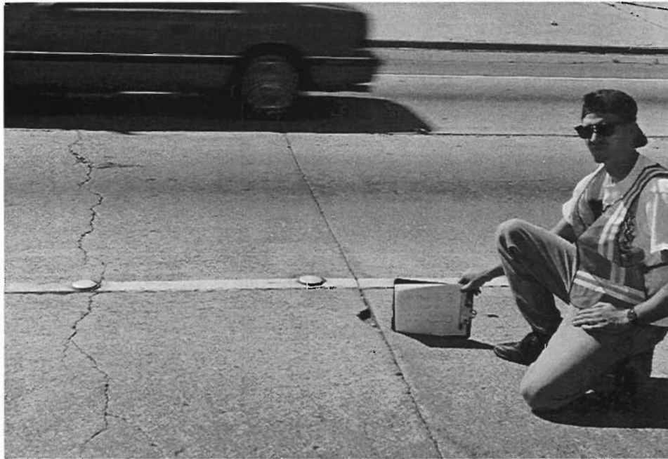
Figure 2.15 Example of spalling on IH-10
