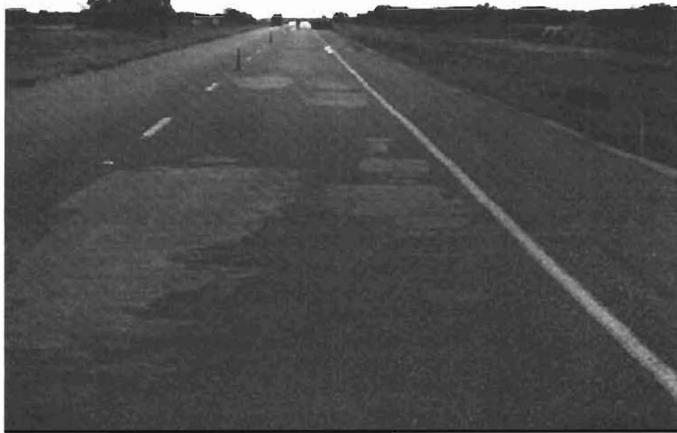
Figure 21. Pavement failure in 4-inch SAS subsection. (View is from south to north.)
