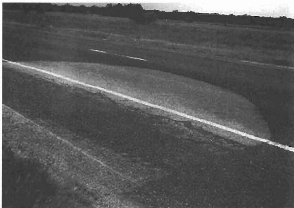
Figure 20. Pavement failure in 10-inch SAS subsection.
