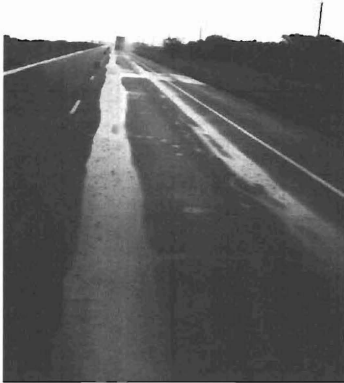
Figure 11. Channelized ponding in 7-inch HMAC subsection. (View is from south to north.)
