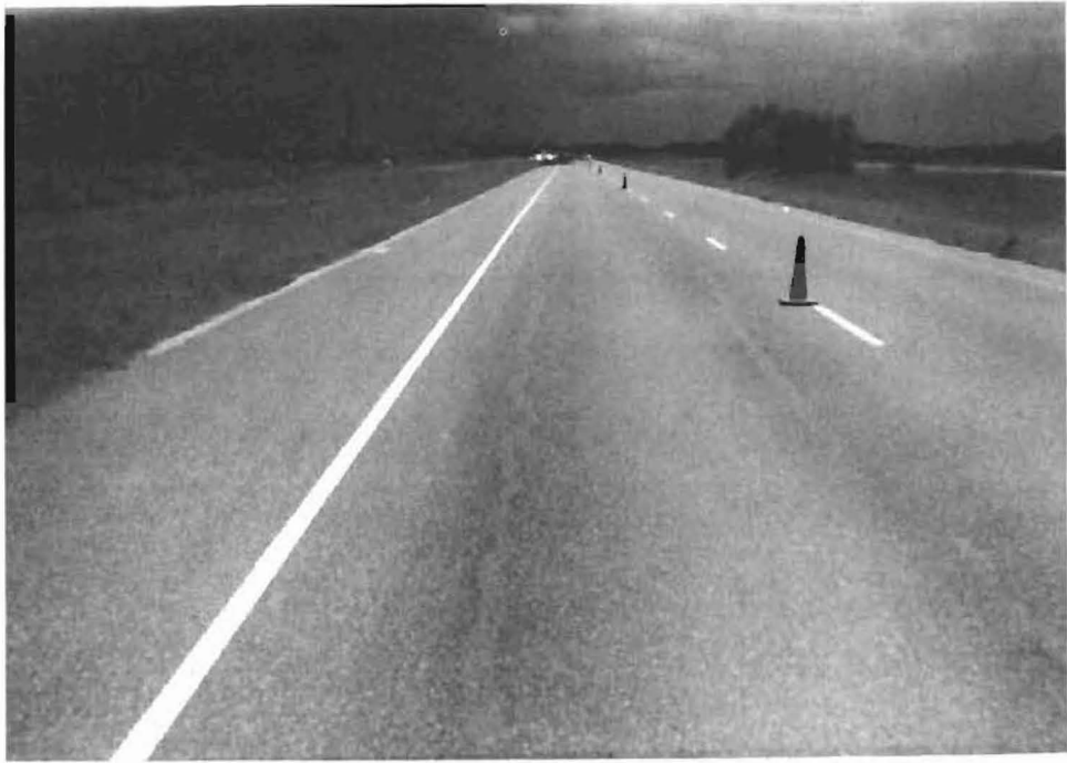
Figure 19. Longitudinal cracking in 4-inch HMAC subsection. (View is from north to south.)
