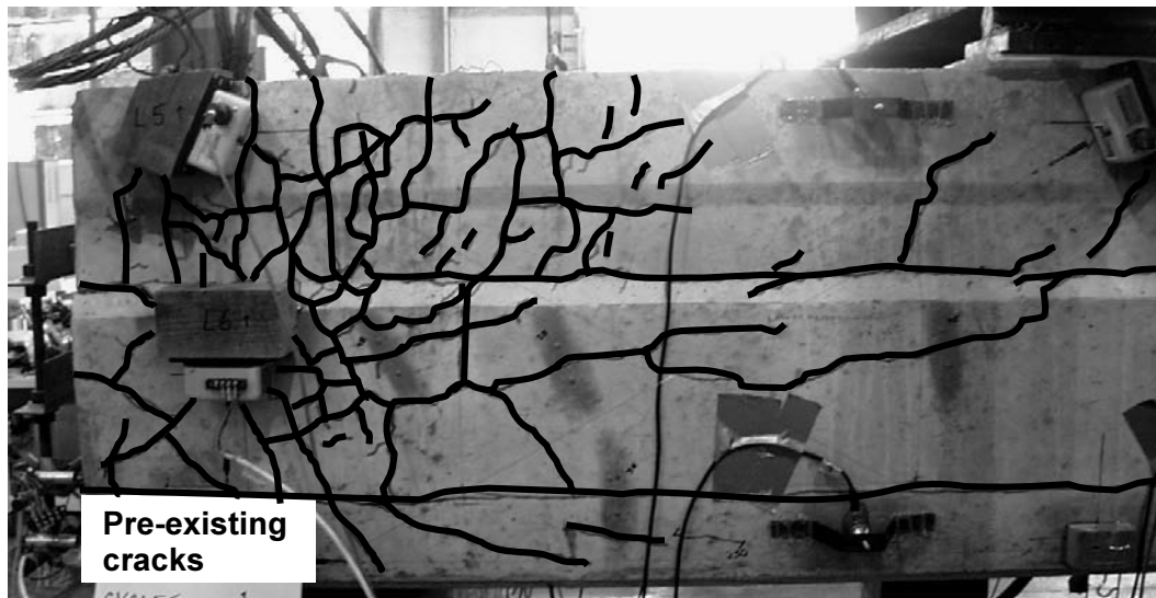
Figure 4.21 Pre-existing cracks in the east web of BG3S
