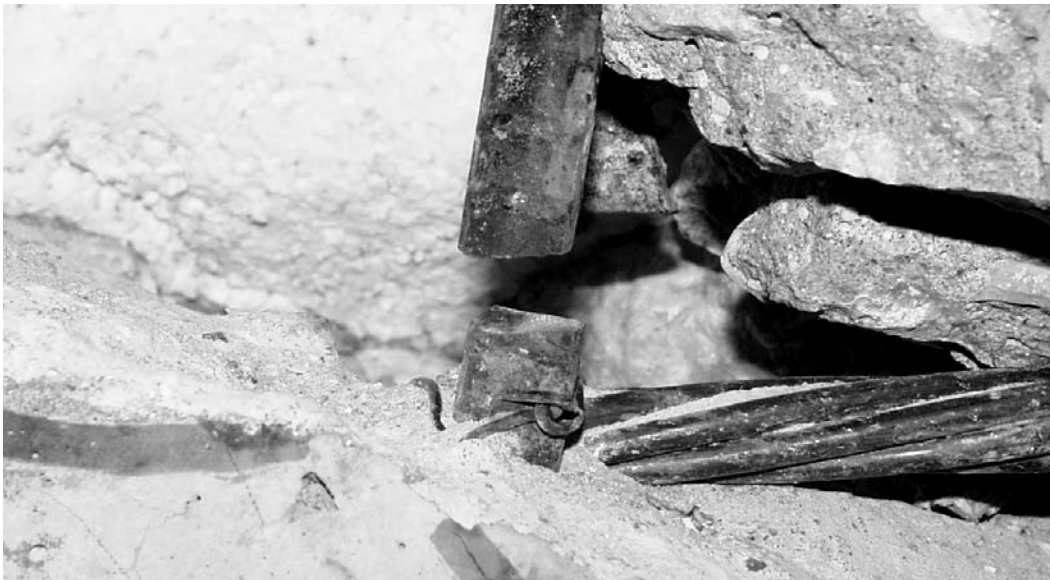
Figure 4.13 Fractured shear reinforcement (stirrup) in the east web of BG3N at failure, after removal of concrete
