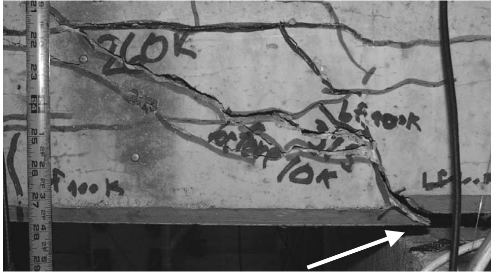
Figure 4.12 Displaced concrete section at the bottom of the east web of BG3N at failure
