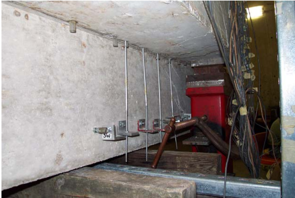
Fig. 2.3(e) LVDTs to study the variation of hanger steel strains along the span
