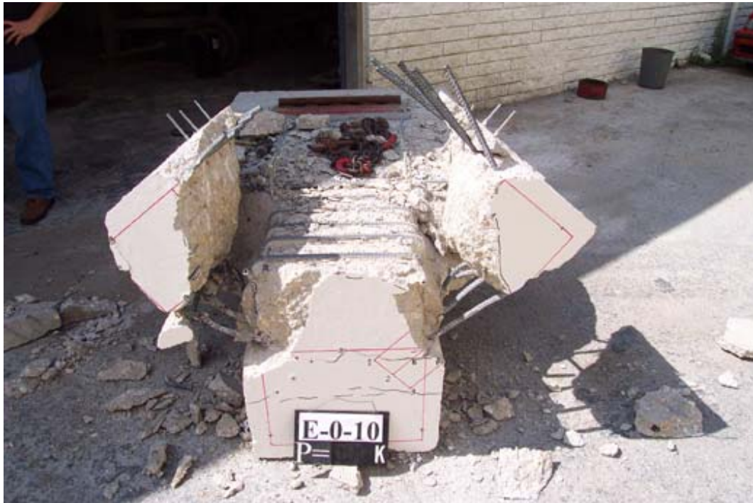
Fig. A9 Punching Shear Failure
