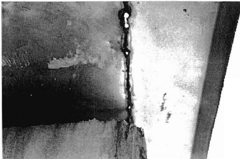
Figure 29 - Retrofitted drip pan, showing poor welding
