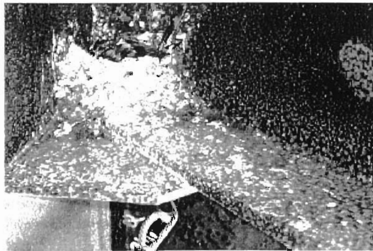
Figure 38 - Accumulated debris completely restricts water flow
