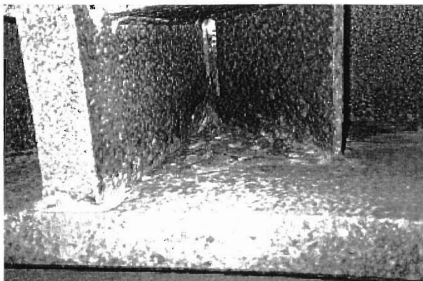
Figure 1 - Gap closure due to inadequately-sized clips
