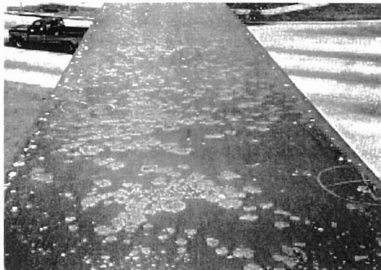
Figure 23 - Incomplete blasting of a steel bent cap
