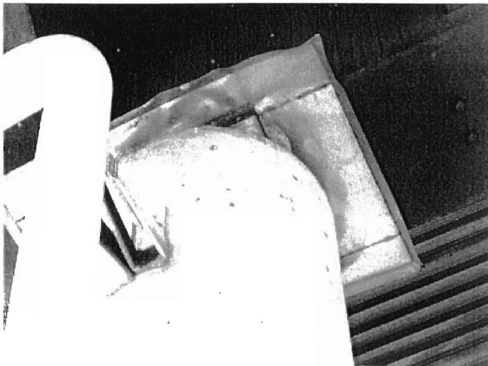
Figure 27 - Properly retrofitted drip pan on pier
