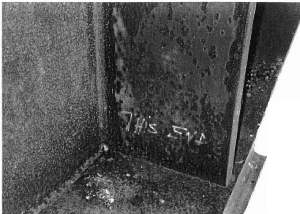
Figure 34 - High Island Bridge stiffener with mill scale still visible
