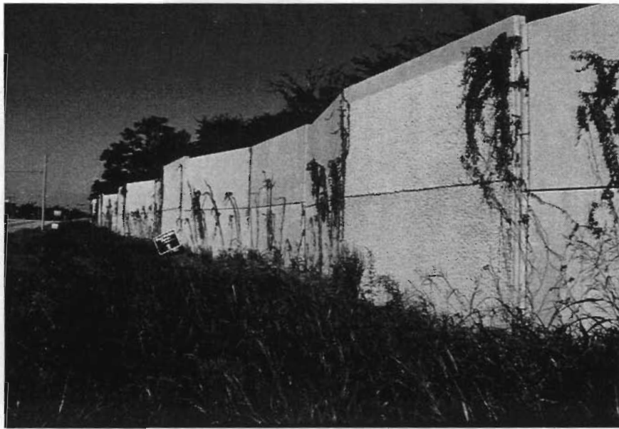
Figure 4.7. Example of Fan-Wall System (Austin District, precast panels interlocked with steel cables)
