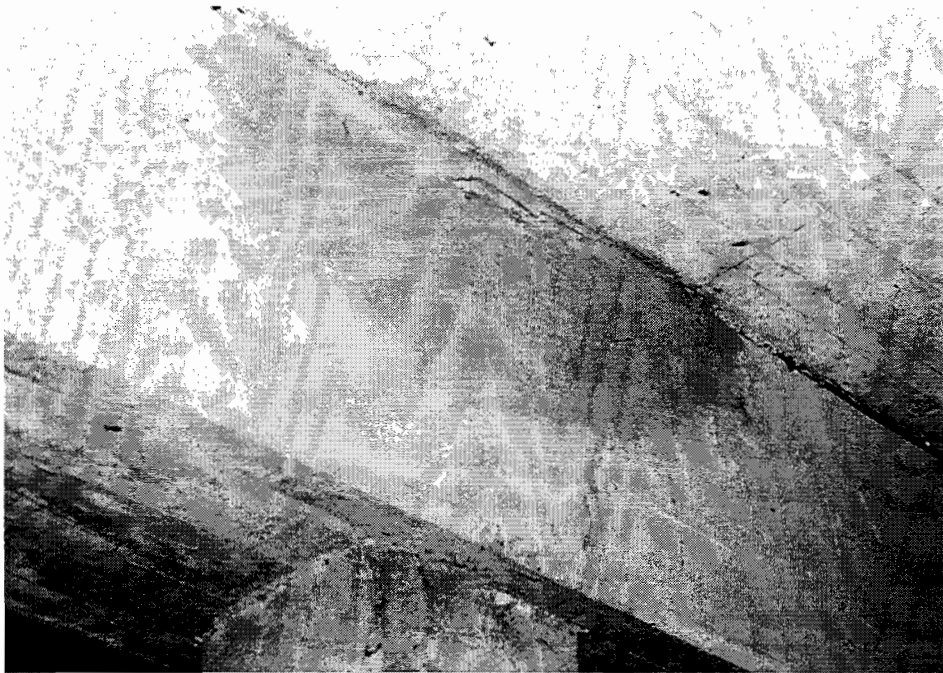
Figure 6.12 Spalling of repaired bent caps — Lufkin No. 2
