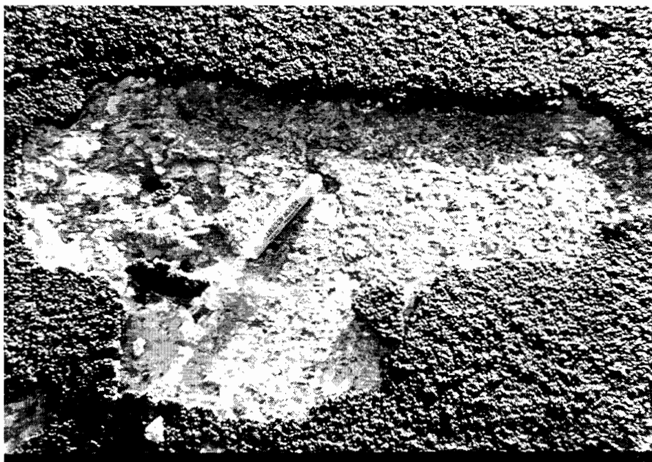
Figure 6.7 Delamination of overlay — Fort Worth No. 1
