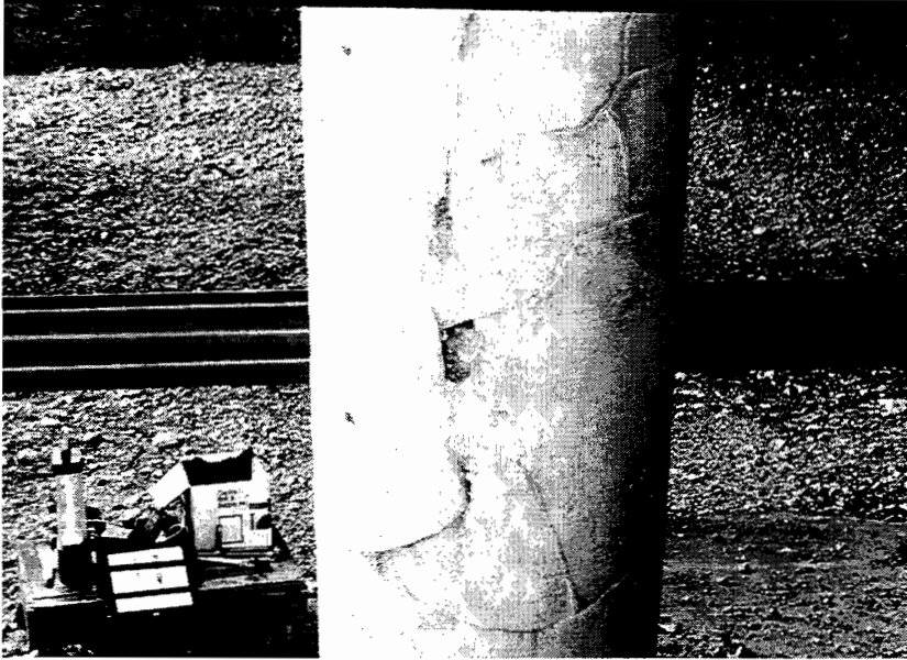
Figure 6.3 Cracking and spalling of repaired column — Austin No. 3
