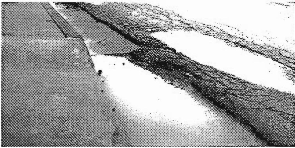
Figure 2.10 Poor Drainage Reduces Traction and Obscures Other Pavement Problems
