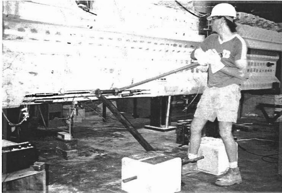
Figure 6-15 Installation of Alberta splice and measurement of average strand elongation to monitor stress level
