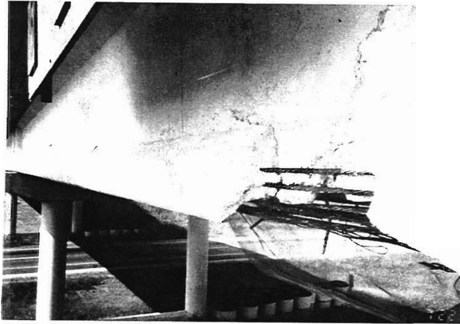
Figure 2-18 Impact damage of Girder 1 — Waelder Bridge
