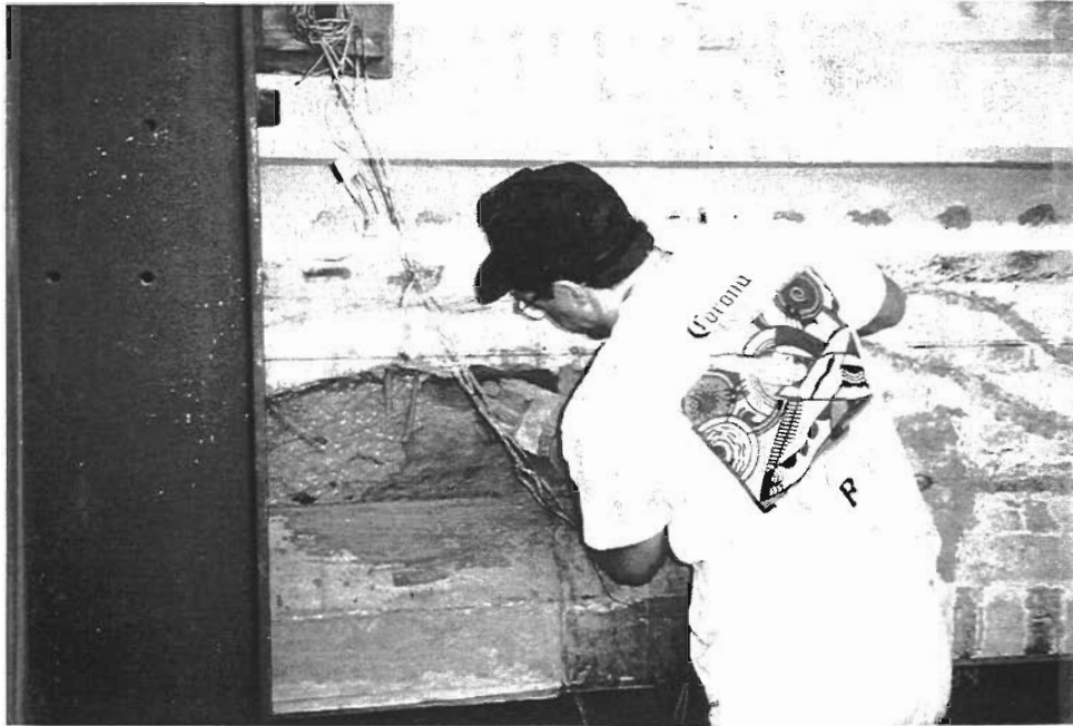
Figure 5- 18 Repair of web damage on impacted side of girder using Burke V/O
