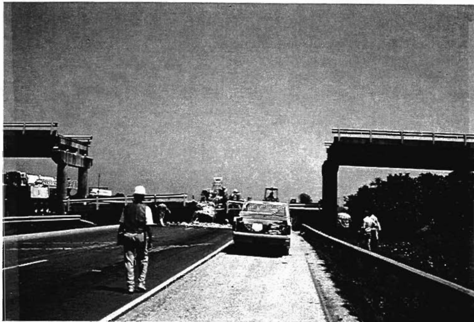
Figure 2-9 Southern view of collapsed structure at Georgetown, Texas
