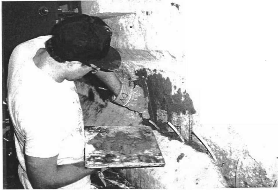
Figure 5- 21 Placement of burke Acrylic Patch on nonimpacted side of girder for repairing damaged area of the web
