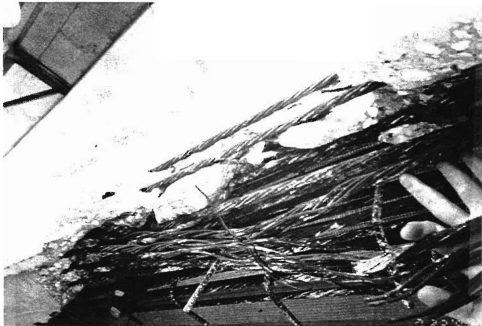
Figure 2-19 Close-up view of damaged strands of Girder 1 — Waelder Bridge
