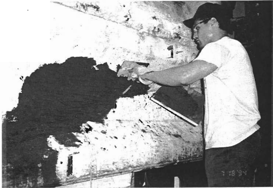
Figure 5- 22 Placement of MasterBuilders Emaco S88CA for web repair of nonimpacted side of girder
