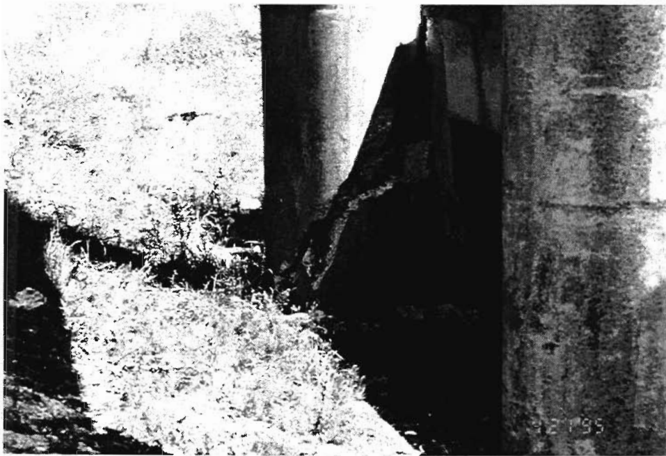
Figure 2- 14 Lodging of collapsed structure against central pier
