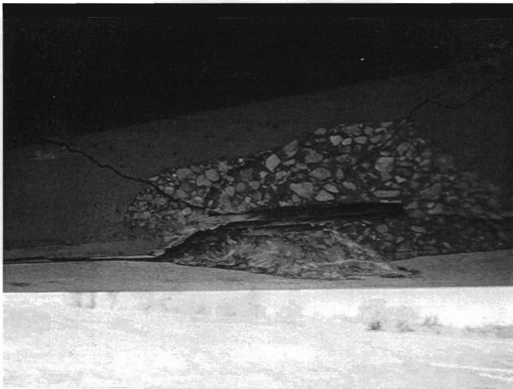
Figure 5- 3 Moderate damage (Courtesy of the Texas Department of Transportation)
