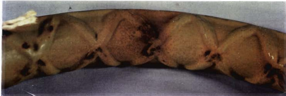
(a) #8 bar with a damage spot > 1/4 in. x 1/4 in. which is < 2%
