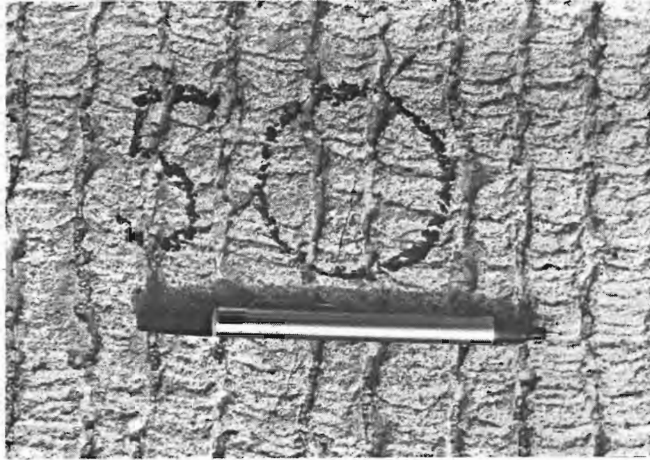
Figure 5.3 A typical crack 0.005 inch wide on BW 8, test section E
