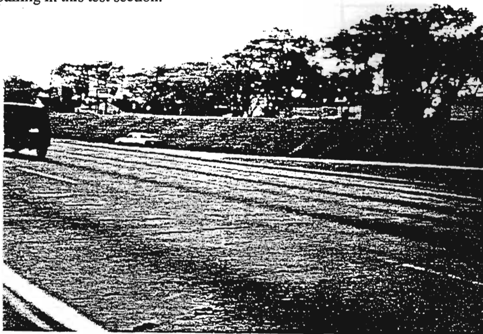
Figure 2.19.1: Spalling in the Westbound Inside Lanes of IH-10 in Houston
