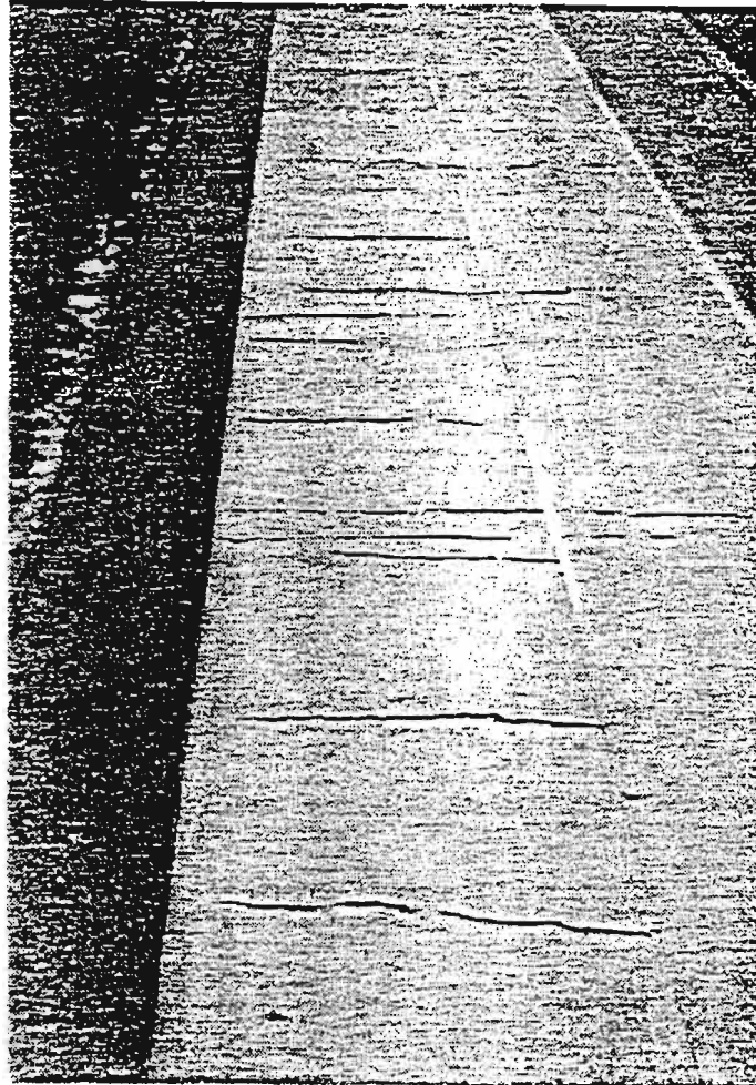
Figure 2.6: Severe Spalling, Inside Lane of SH-6 Bypass, District 17, Brazos County
