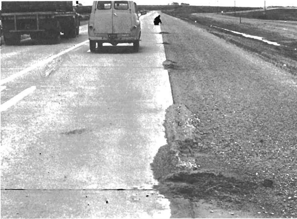
Fig 6. Typical quantities of granular subbase material (maximum size 1\frac{1}{2} " ) pumping from beneath portland cement concrete panel at the AASHO Road Test.
