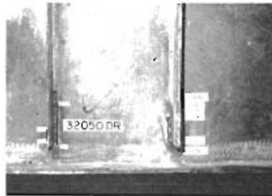
OVERALL VIEW OF THE CRACK
