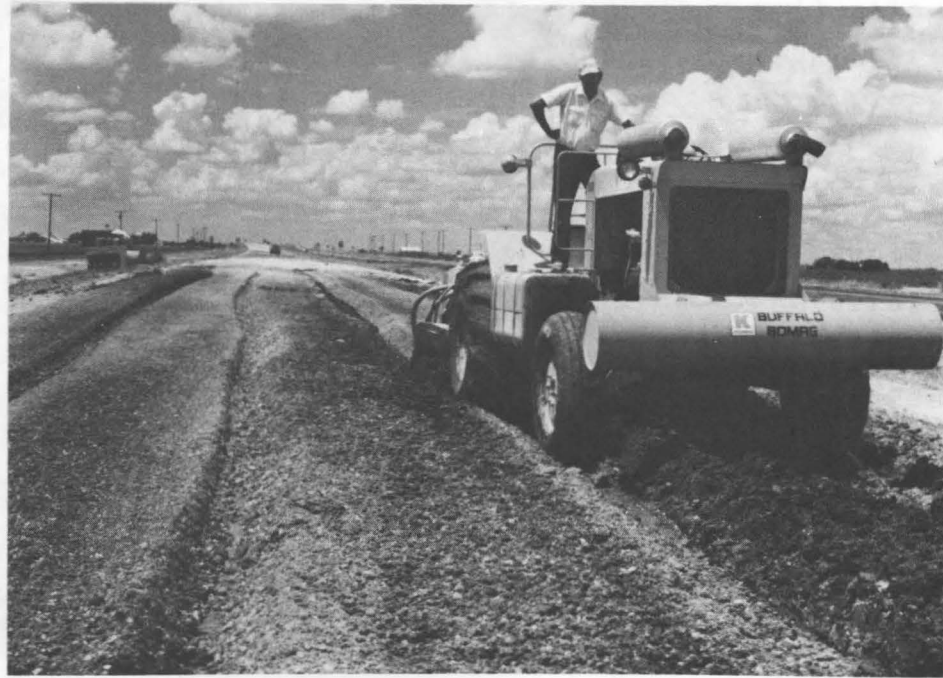
Picture #3 - High speed mixer used to mix emulsion into existing base material.
