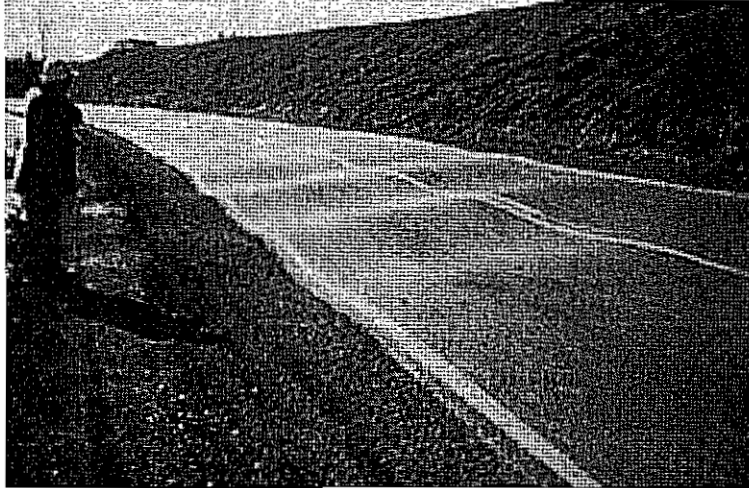
Figure 2.4 - Pavement Damage Due to Frost Heave (www.tfhrc.gov)
