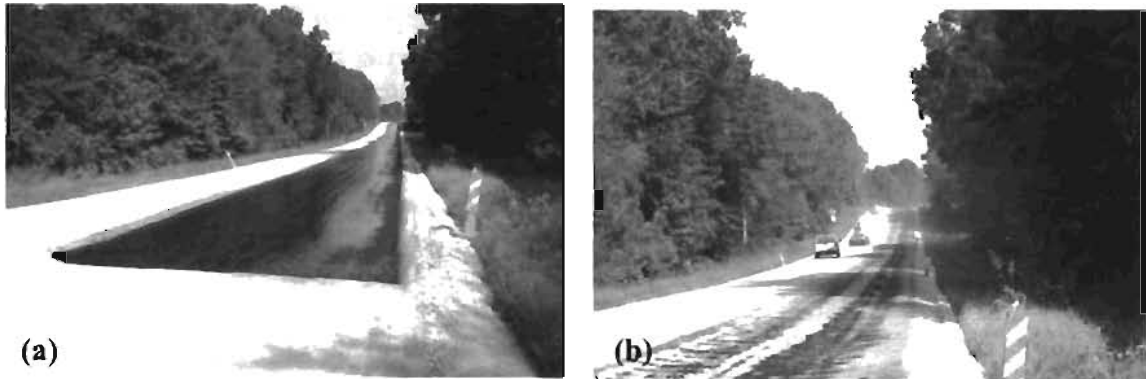
Figure 3.2 Spray Prime (a) MC-30 Cutback Prime (b) Blotting Sand Applied on Prime
