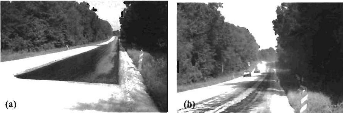
Figure 6 Spray Prime (a) MC-30 Cutback Prime (b) Blotting Sand Applied on Prime
