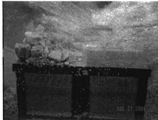
Figure 11. Deposition on top of culvert.
