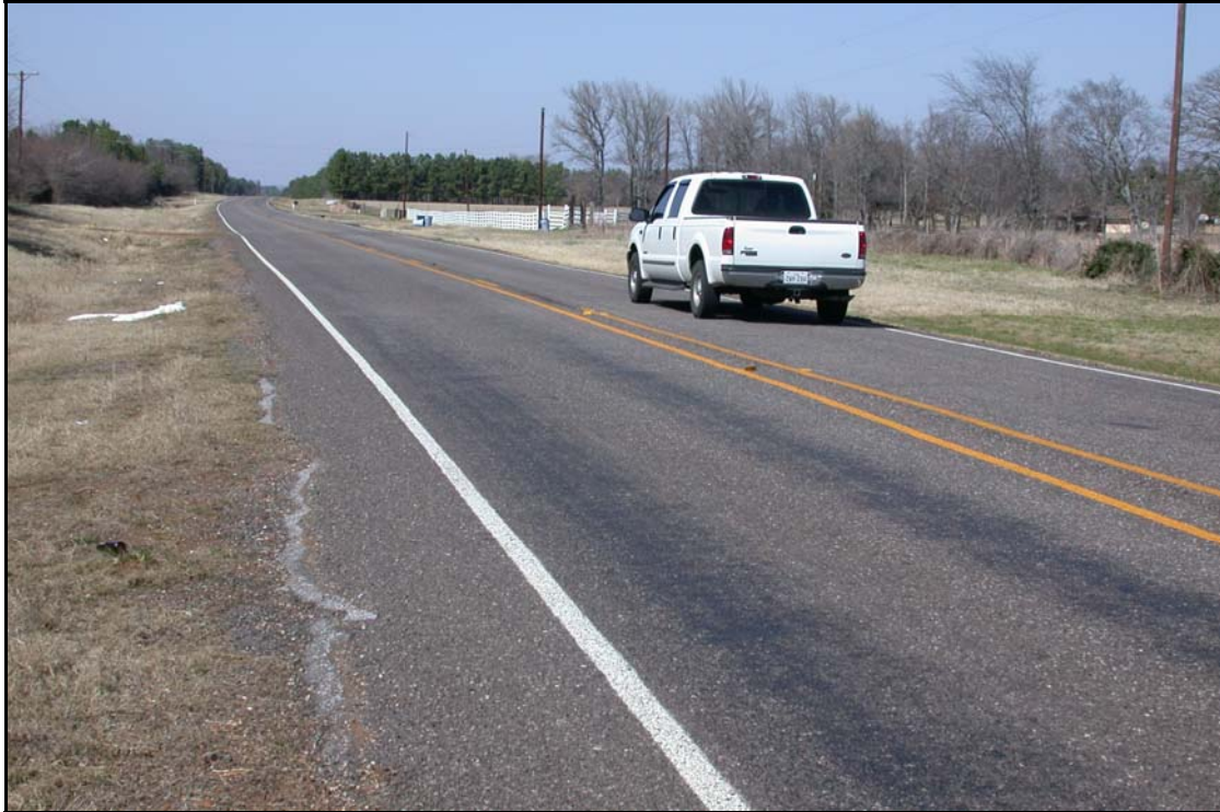
FIG. 6.19. FM 2661 Road Widening, Smith County Texas, Tyler District (see Tyler District Profile, Photo 8)
