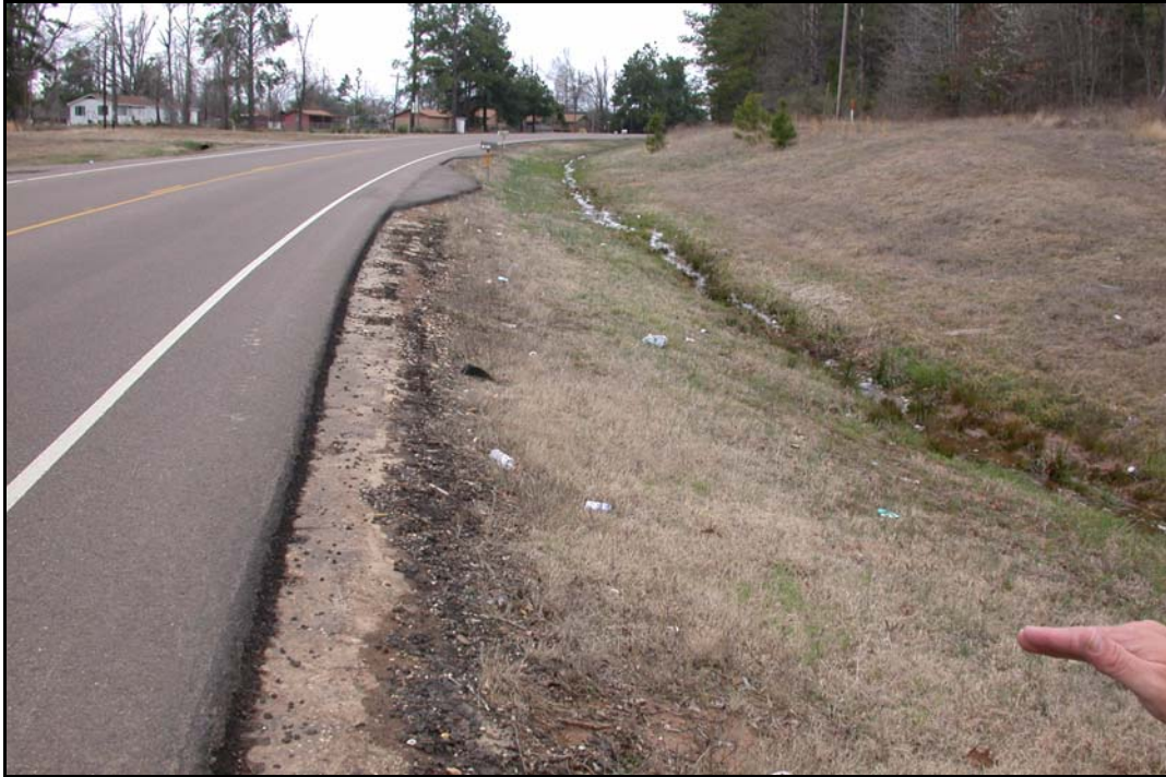
FIG 5.13 Erosion-induced Edge Drop-off Following an Overlay, Atlanta District (see Atlanta District Profile, Photo 11)
