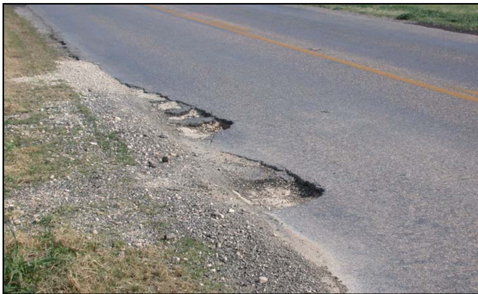
FIG 5.22 Fishmouth-type Edge Failure, San Antonio District (see San Antonio District Profile, Photo 12)
