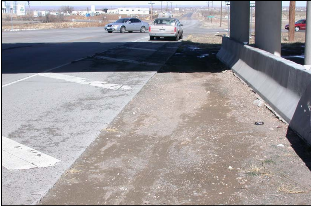
FIG. 4.16. Pavement Edge Damage Associated with Vehicle Pull-offs Beneath an Overpass.
