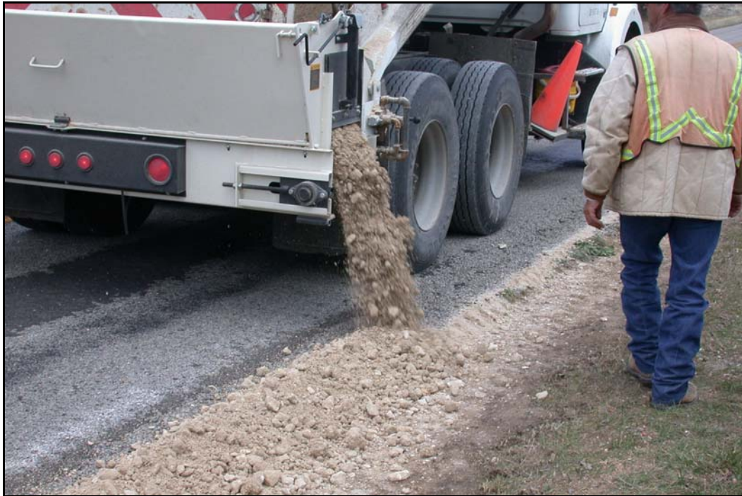
FIG. 5.27 Delivering Flex Base to the Pavement Edge Using a Swenson Tailgate Cross Conveyor (a.k.a. “Swenson Spreader”), Brownwood District (see Brownwood District Profile, Photo 13)
