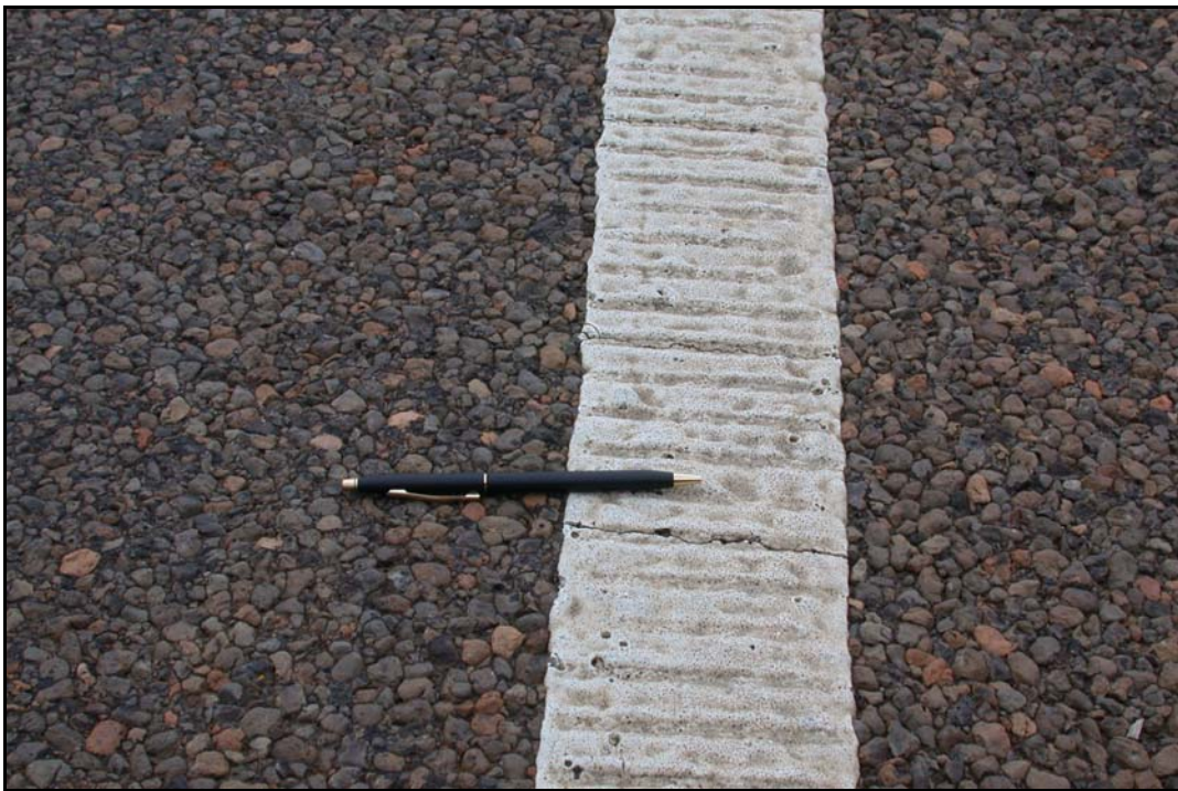
FIG 5.21 Inverted Profile Pavement Marking, Close-up View, Atlanta District (see Atlanta District Profile, Photo 26)
