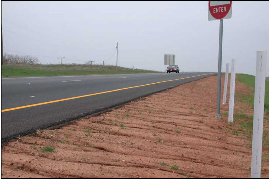
FIG 5.6 Soil Erosion of Pavement Edge Backfill due to Improper Specification, Wichita Falls District (see Wichita Falls District Profile, Photo 7)
