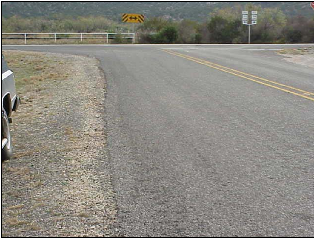
FIG 5.11 Intersection Approach Apron, San Angelo District (see San Angelo District Profile, Photo 5)
