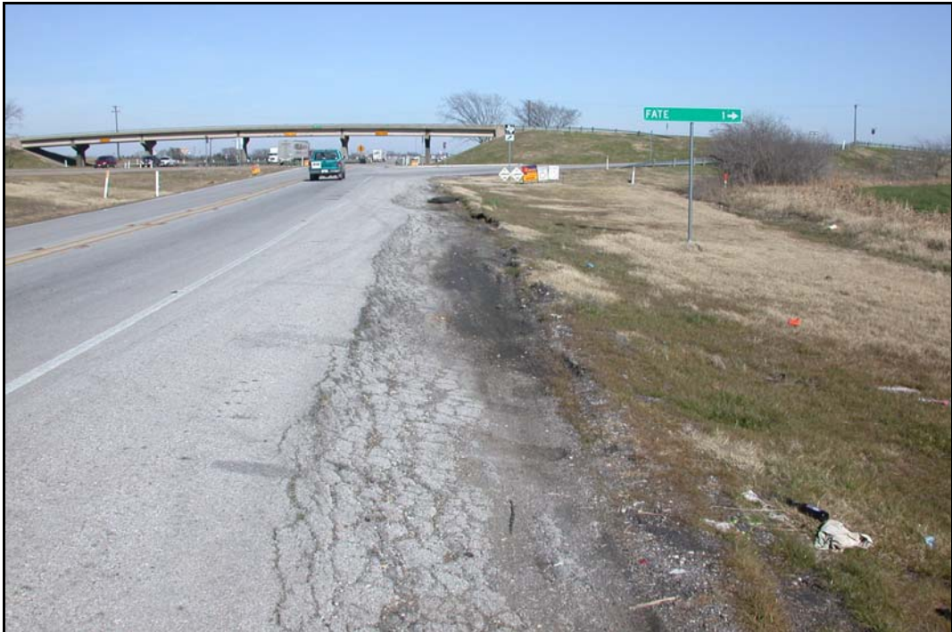
FIG. 4.10. Edge Damage Along Interstate Highway Access Road.
