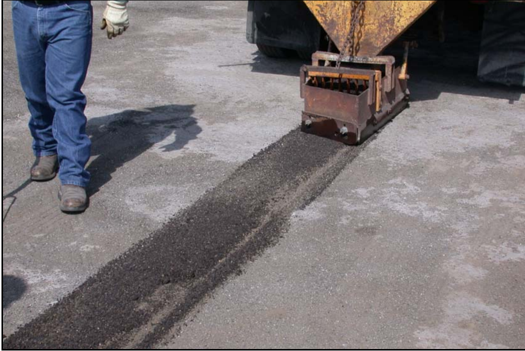
FIG. 5.33 Limestone Rock Asphalt (LRA) for Pavement Edge Repair, Pharr District, (see Pharr District Profile, Photograph 7)
