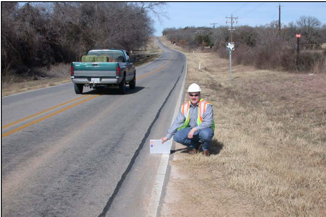
FIG. 6.18. FM 113 Road Widening, Parker County Texas, Fort Worth District (see Fort Worth District Profile, Photo 23)
