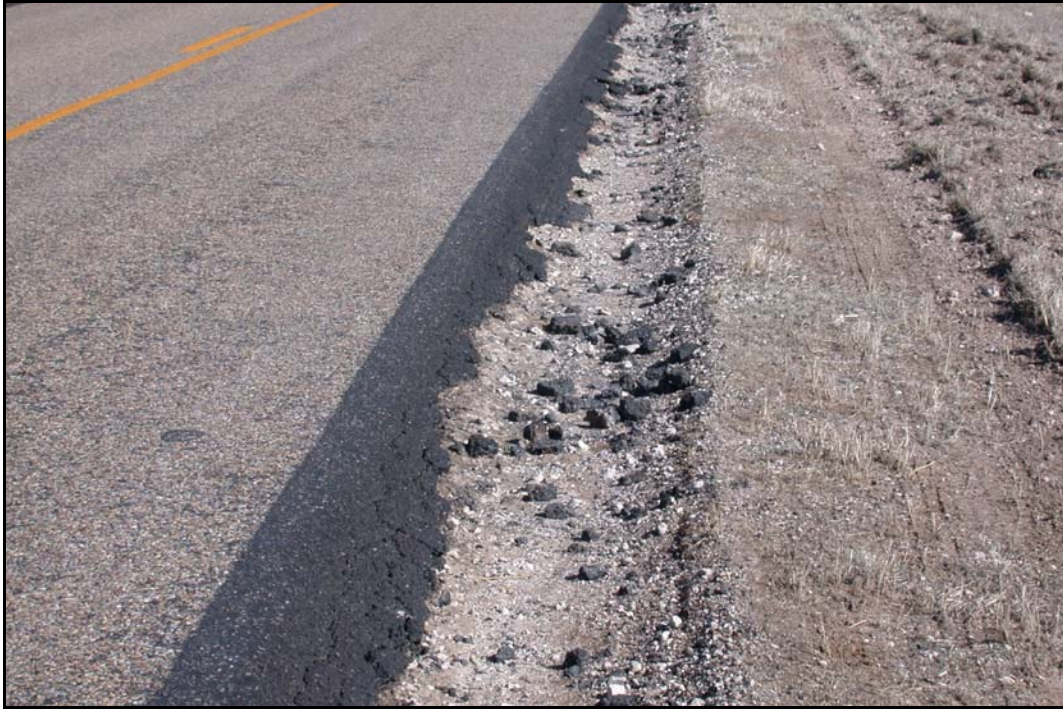
FIG. 4.22. Typical Edge Damage on a Low Volume Road Caused by Snow Plow Operations.
