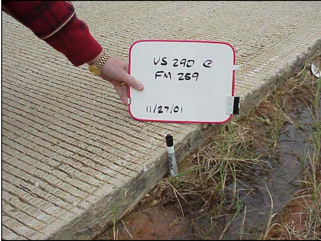
FIG. 4.26. Edge Drop-off Associated with Wet Subgrade Along the Edge of Pavement
