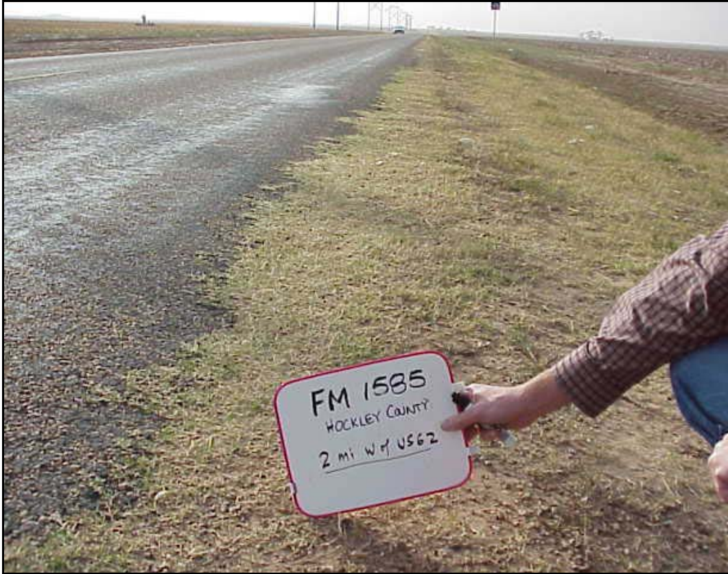
FIG 5.15 Encroachment of Vegetation onto the Pavement Edge, Lubbock District (see Lubbock District Profile, Photo 16)
