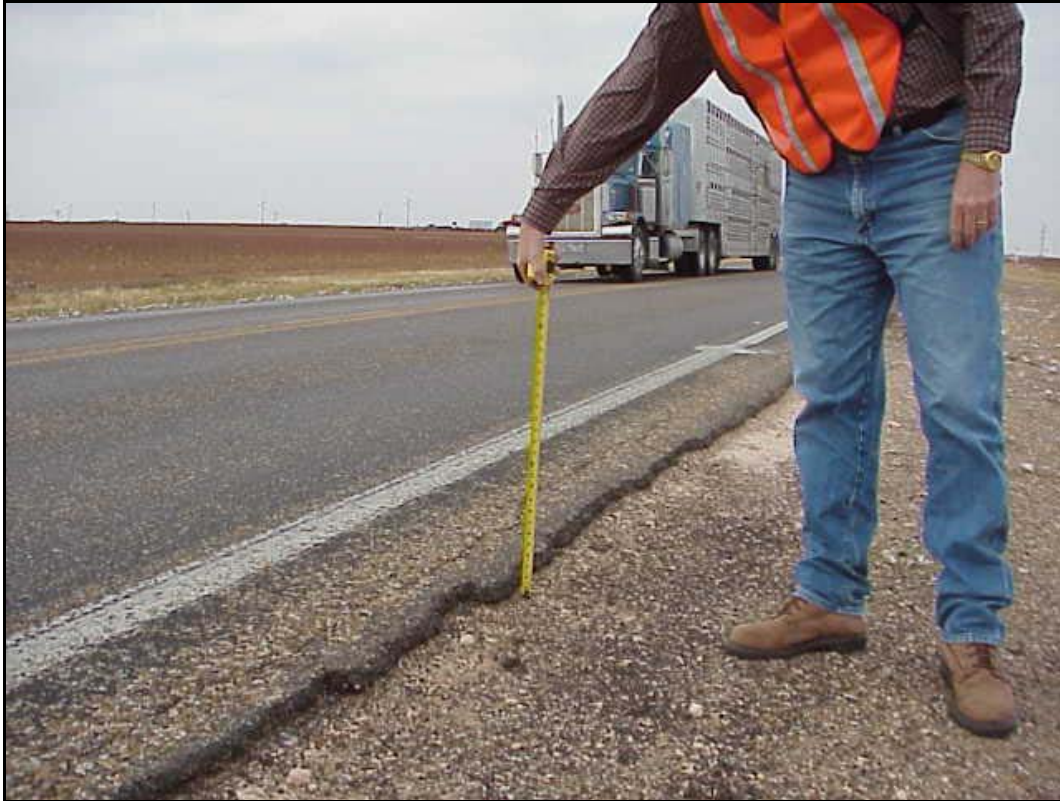
FIG. 4.15. Typical Pavement Edge Damage Associated with Cotton Production in West Texas.
