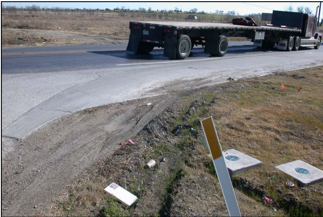
FIG. 4.20. Edge Damage Caused by Cutting Corners at a Convenience Store Access Drive.
