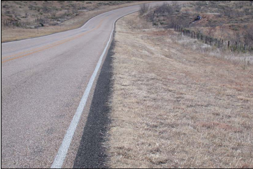
FIG 5.9 Raw Edging, Amarillo District (see Amarillo District Profile, Photo 9)
