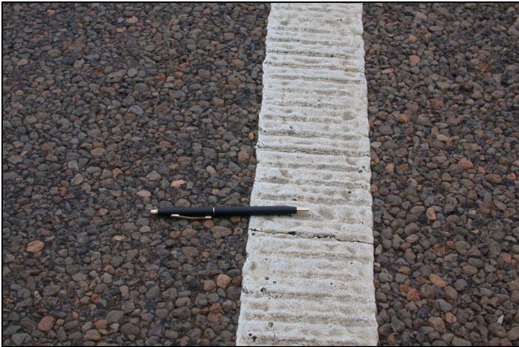
FIG 5.21 Inverted Profile Pavement Marking, Close-up View, Atlanta District (see Atlanta District Profile, Photo 26)
