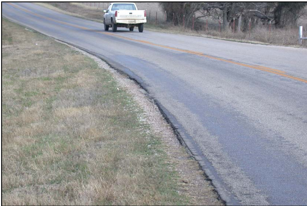
FIG. 4.11. Typical Edge Drop-off at Inside Horizontal Curve on a Low Volume FM Road.
