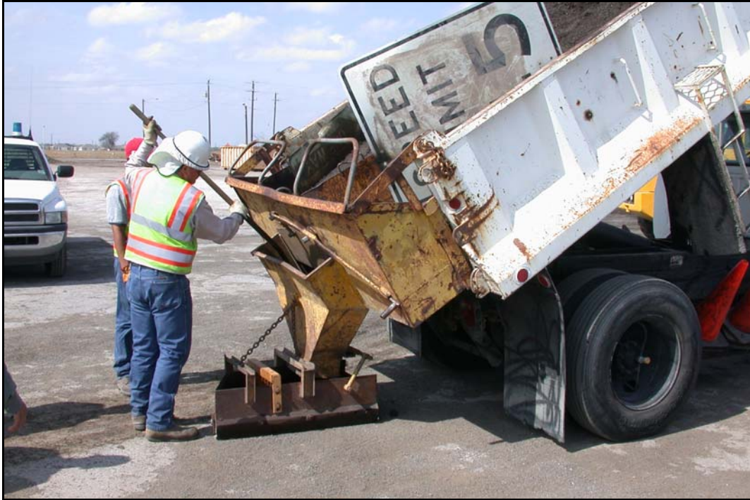
FIG. 7.11 Center-Discharge Tailgate Chute with Drag Box, Pharr District (see Pharr Profile, Photos 3 through 5)
