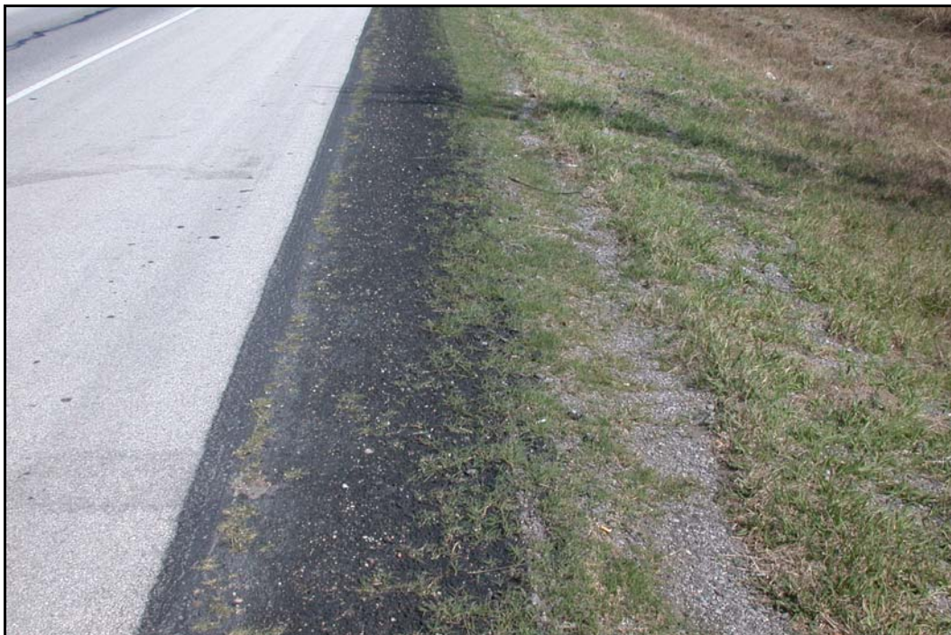
FIG 5.14 Edge Seal to Promote Vegetation Growth, Yoakum District (see Yoakum District Profile, Photo 7)
