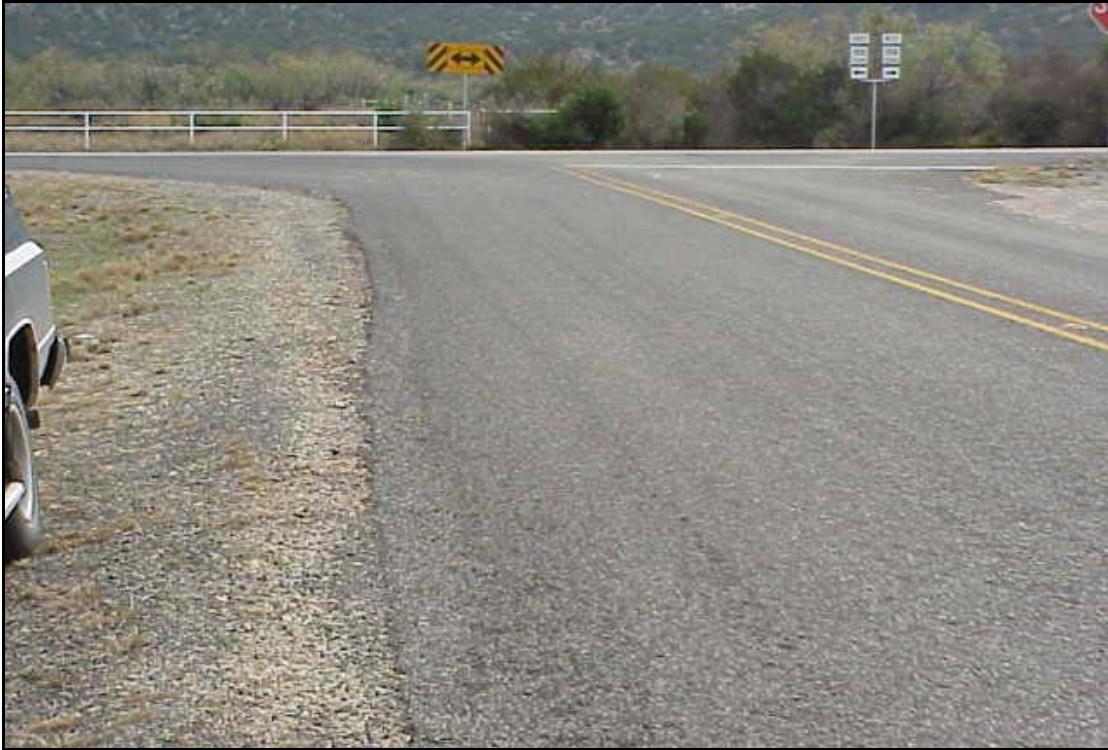
FIG. 6.13. RM 2059 Road Widening, Coke County Texas, San Angelo District (see San Angelo District Profile, Photo 14)
