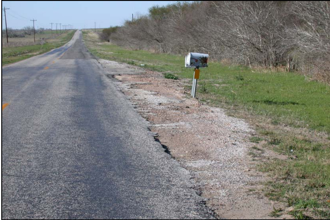
FIG. 4.14. Typical Edge Drop-off at Mail-box Turnout.
