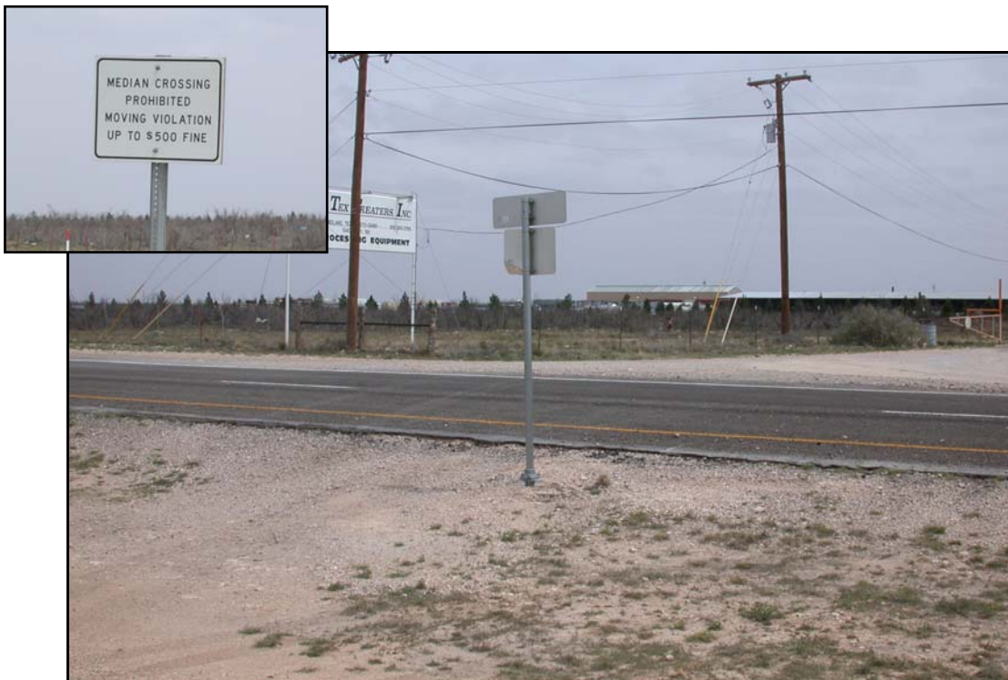
FIG. 4.17. Pavement Edge Damage Associated with Illegal Median Crossing. The Inset Shows the Regulation Sign Posted Where the Crossing Continues to Occur
