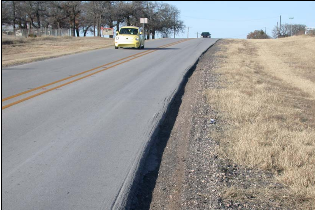
FIG. 4.8. Edge Drop-off at Relatively High-Volume, Narrow FM Road (21-foot width, ADT 4,400 vehicles/day).
