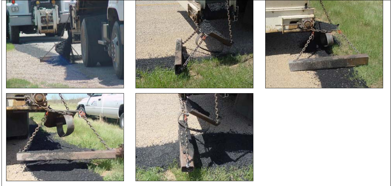
FIG. 7.15 Photo Series: Side Discharge Chute and Tow-Behind Drag Bar for Edge Repair, Wichita Falls District
