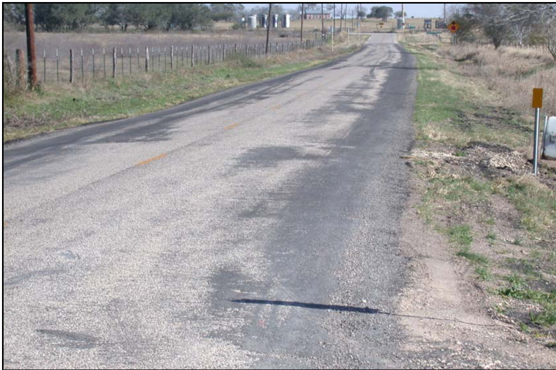
FIG. 6.14. FM 239 Road Widening, DeWitt County Texas, Yoakum District (see Yoakum District Profile, Photo14).
