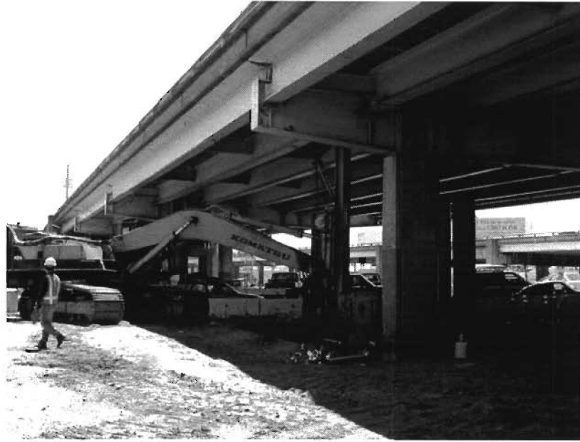
Figure 5.6 Use of Limited Headroom Pile Driver in the Retrofit of Pier Foundations in the San Francisco-Oakland Bay Bridge (Source: bbuckland@mandelpipe.com )
