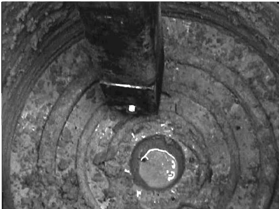
Fig. A.1.2 Static Penetrometer Mounted on Kelly Being Pushed by Weight of Kelly at the Bottom of a Drilled Shaft Borehole
