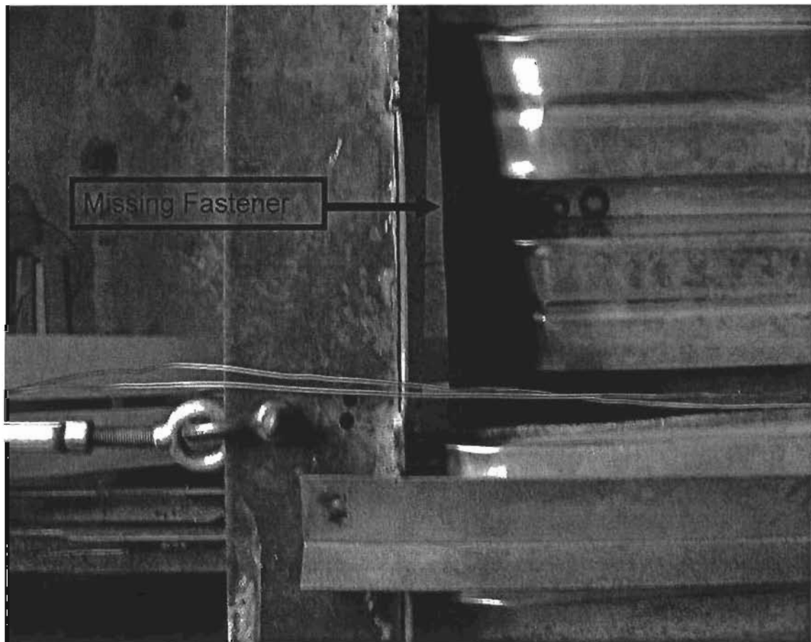
Figure 7.39 Photo of Failure of the Deck to Support Angle Connection
