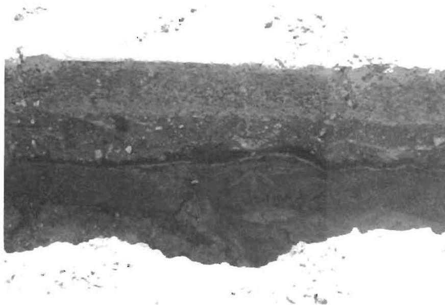
Fig 4.9. Lenses of grout at the interface between CTB and the Subgrade Clay material.
