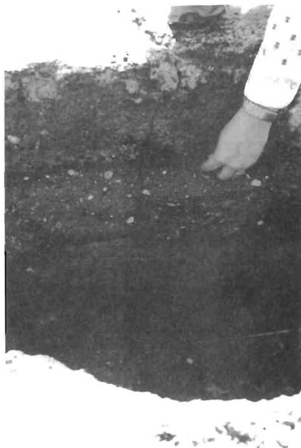
Fig 4.8. Punchout crack going through the CTB.
