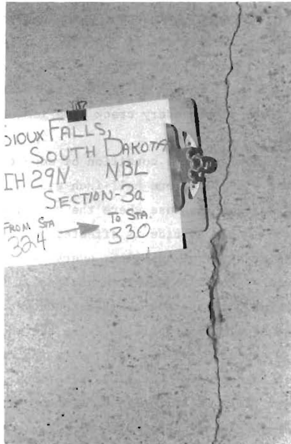
Fig B.5. Minor spalling.
