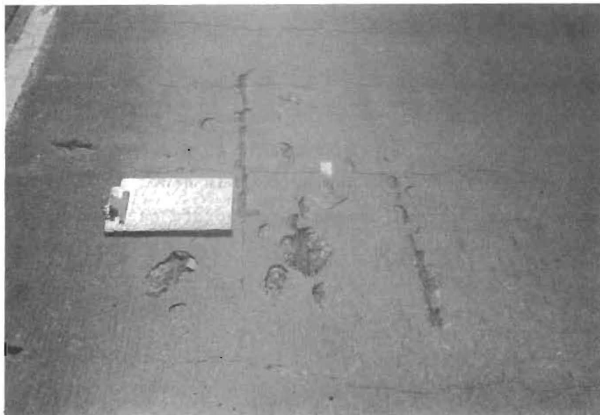
Fig B.17. Steel reinforcement too close to surface.
