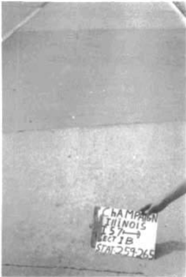
Fig B.13. Portland cement concrete patch defined as severe.
