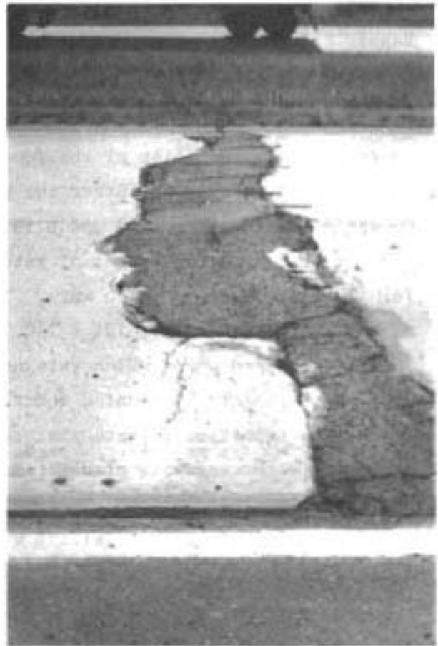
Fig B.12. Asphaltic concrete patch defined as minor.
