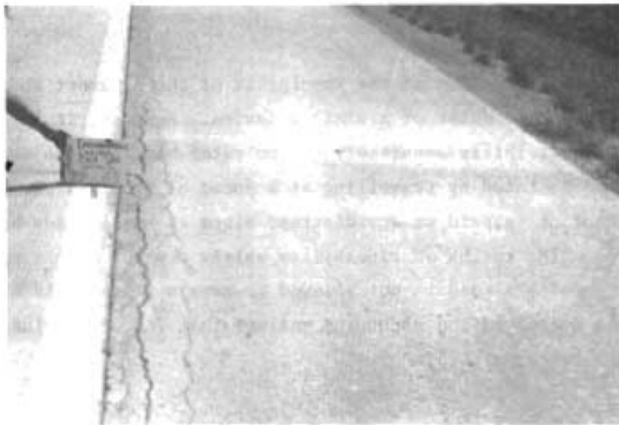
Fig B.14. Shoulder distress, open joint with cracking.
