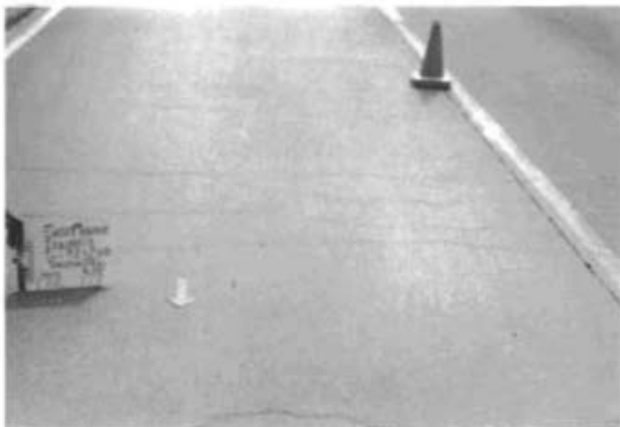
Fig B.3. Minor localized cracking.
