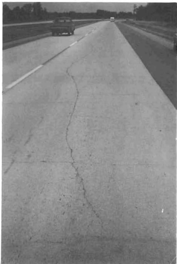
Fig B.9. Longitudinal cracking not to be rated.
