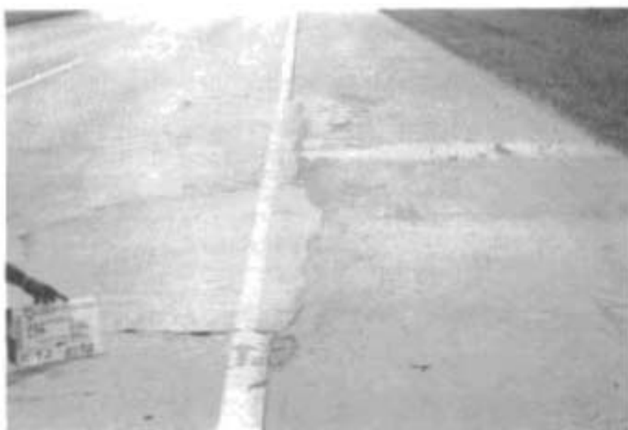
Fig B.8. Severe pumping.
