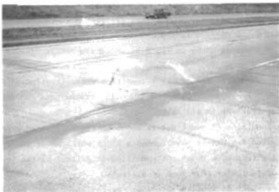
Fig B.7. Minor pumping.
