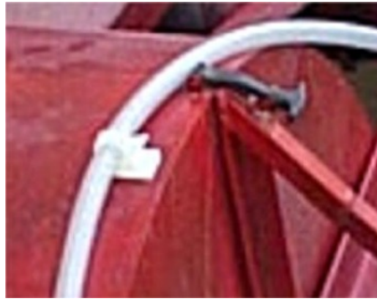
Figure 4-14. Hose Clamp and Fender Hold Down Close up
