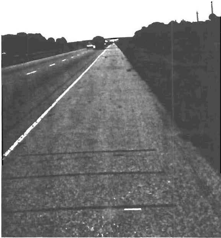
Fig. 2.5 Raised cold mix rumble strips in groups of three with approximately 100 ft (30.5 m) spacing between 3-strip groups.
