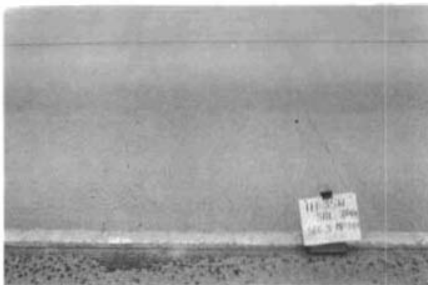
Fig A3.7 Desired transverse crack spacing of from 5 to 8 feet, performance is good, Johnson County.
