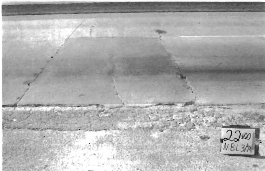
Fig A3.2 PCC repair patch with a transverse crack, Falls-McLennan Counties.
