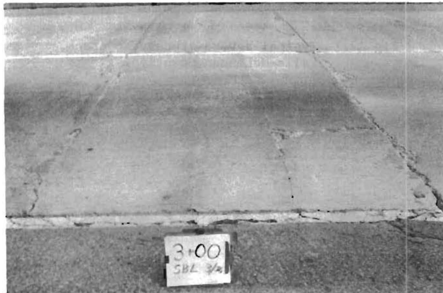
Fig A3.4 PCC repair patch with a punch-out failure, Falls-McLennan Counties.
