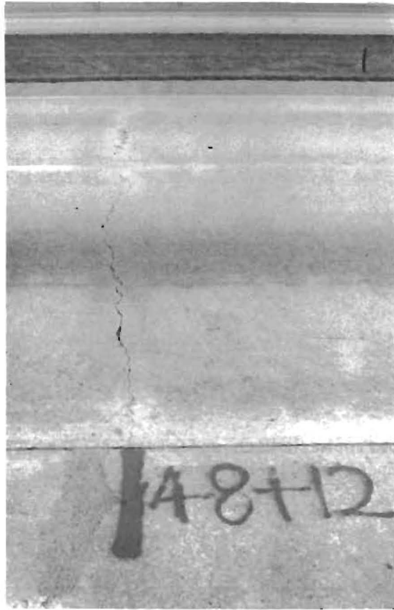
Fig A3.1 Typical severe transverse crack, Falls-McLennan Counties.
