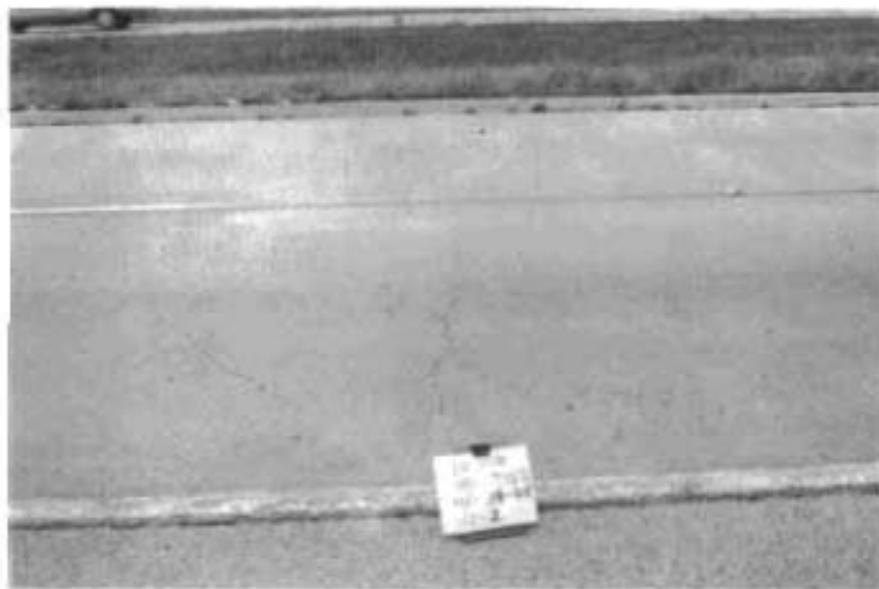
Fig A3.9 Y-cracking (minor), Johnson County.
