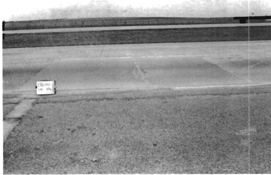
Fig A3.3 PCC repair patch with an interior transverse crack which has pumping, Falls-McLennan Counties.
