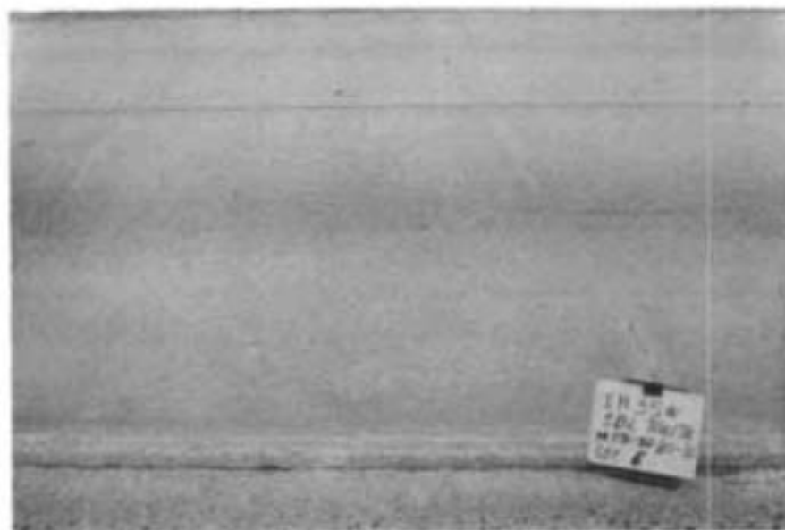
Fig A3.8 Desired transverse crack spacing of from 5 to 8 feet, performance is good, Johnson County.
