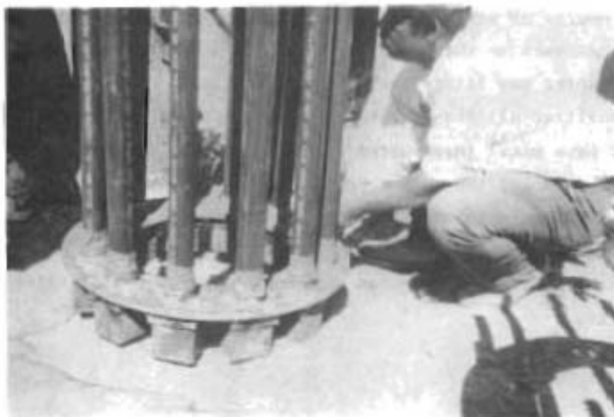
Fig 6.12. Plastic tube pushed into the steel stub and cloth tape wrapped around it.
