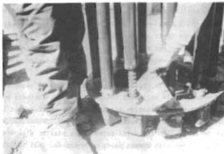
Fig 6.11. Molten wax being poured into the steel stub around the DYWIDAG bars.
