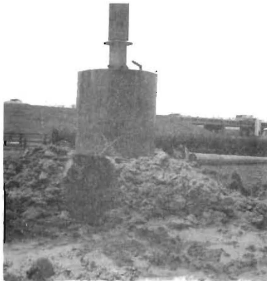
c. Bucket Cleaning of the Bottom of a Hole Drilled Under Mud
