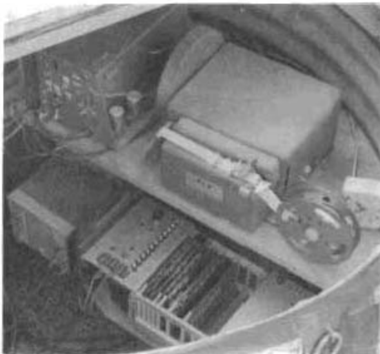
Fig 4.4. Interior and exterior view of instrument shelter.
