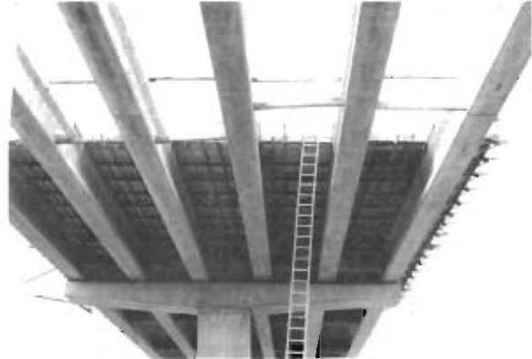
(b) Formwork in progress with only one diaphragm (at one end of the span) cast
