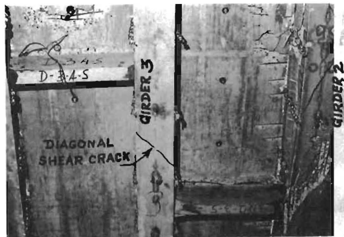
(c) Diagonal crack in Girder 3 due to impact on Girder 2, with diaphragms at 1/3 points of the span
