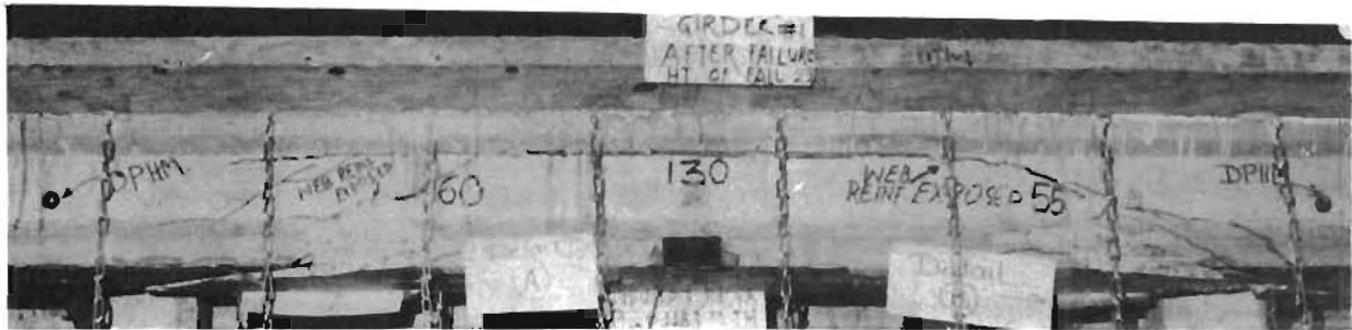
(a) Girder 1 after failure, with diaphragms at 1/3 points of the span (height of fall = 29 in.)
