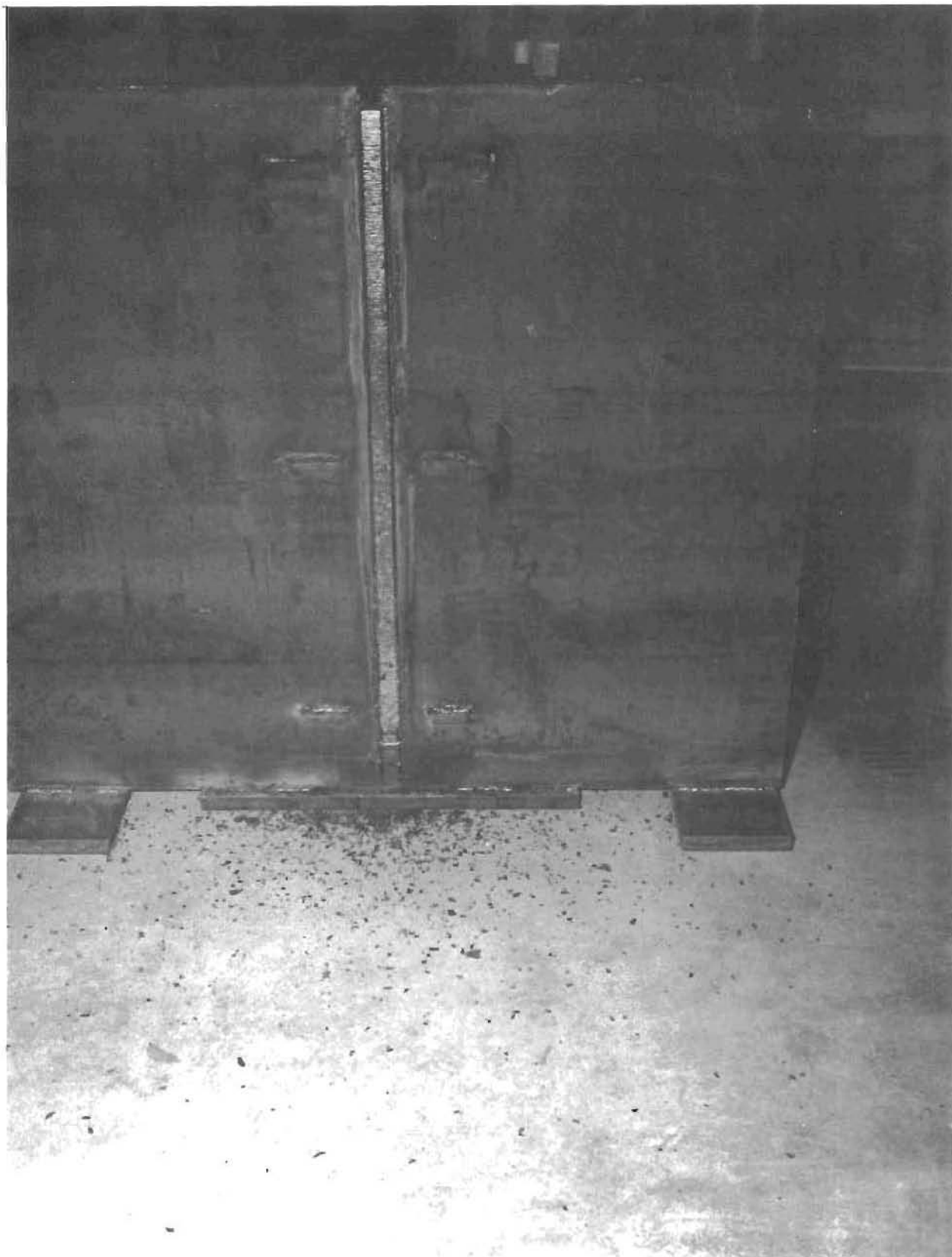
Fig 18. Weldment at end of welding operation. Notice discontinuity near bottom where welding was temporarily halted.
