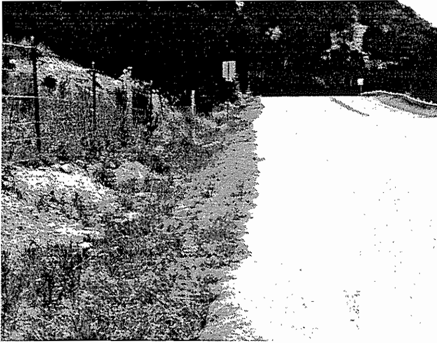
Figure 6.7: Uneven terrain between the pavement and right of way
