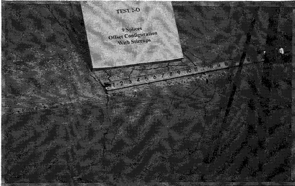
Cracking of side cover
