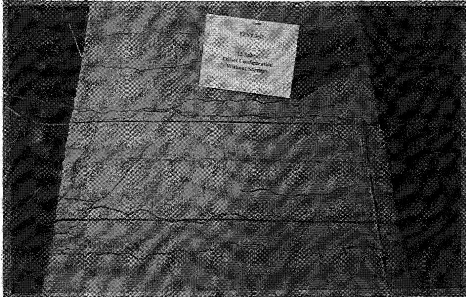
Cracking of face cover
