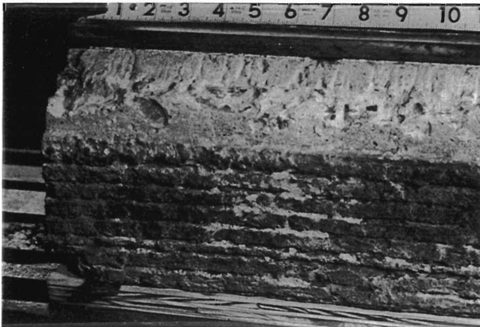
Figure 45 The oval at the left near 2-in. shows a void underneath the rail
