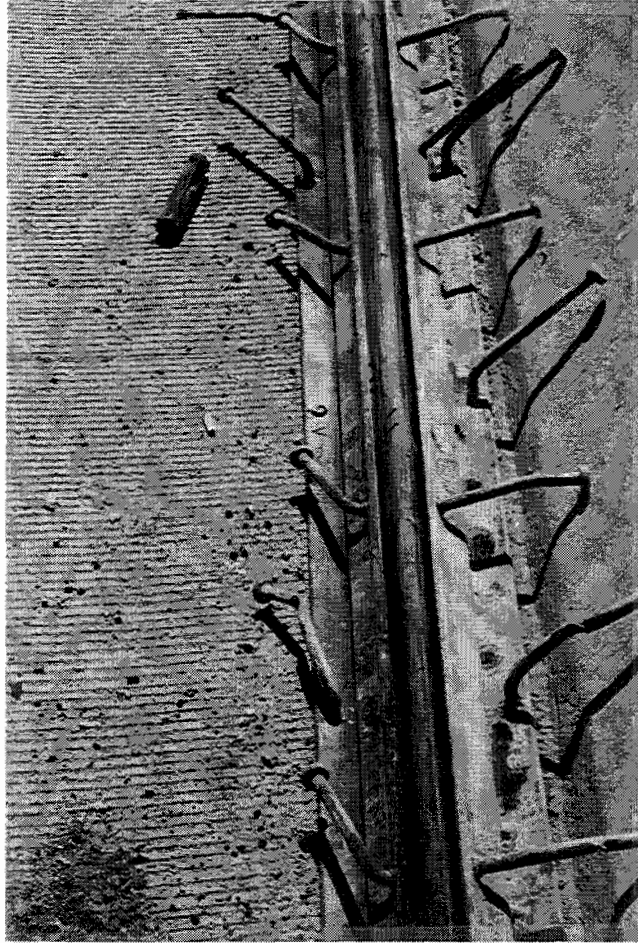
Figure 4 Left side of rail shows several bent over studs without failure
