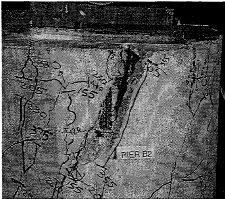
Figure 3.14 Opening of Flexure/Shear for Pier B-2 - Spalled Cover Removed
