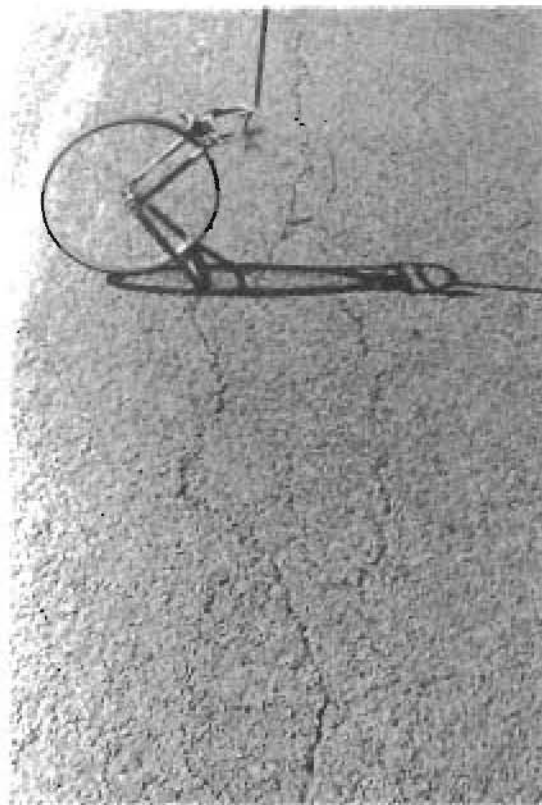
(h) Longitudinal shrinkage cracking.
