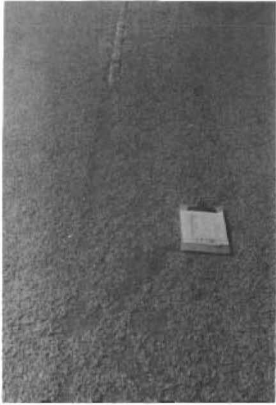
(l) Raveling of aggregate.
