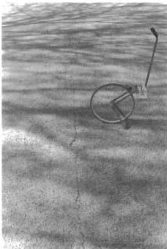
(c) Longitudinal construction crack.
