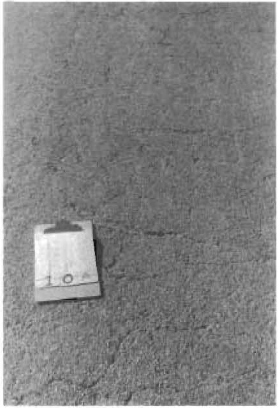
(k) Block cracking.
