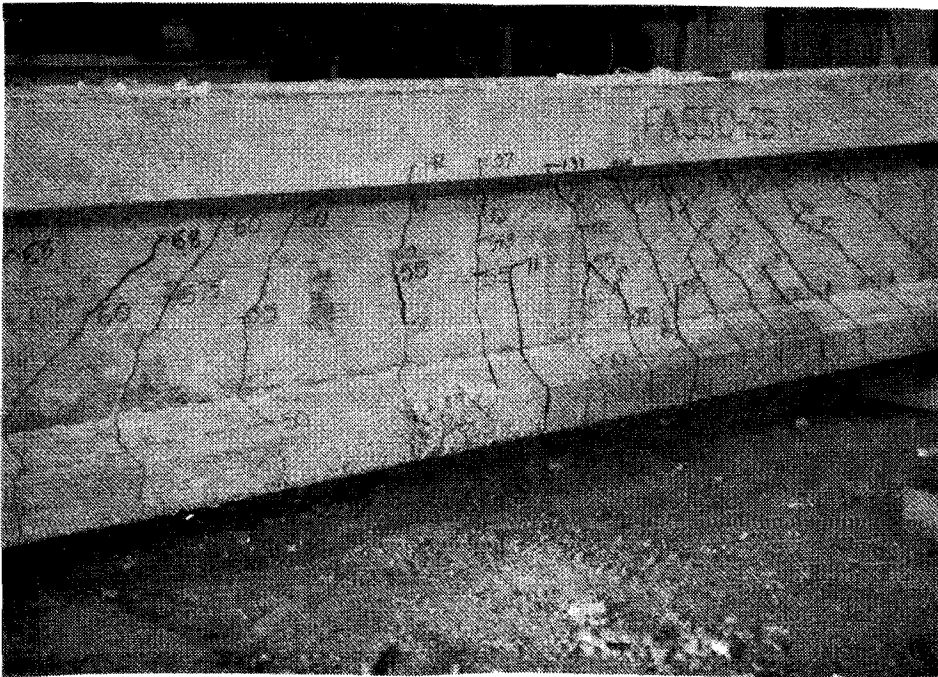
Figure 4.7 Crack pattern for FA550-2B.
