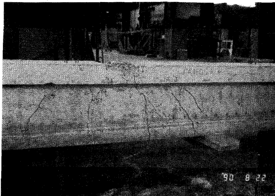
Figure 4.8 Crack pattern for FA460-2A.
