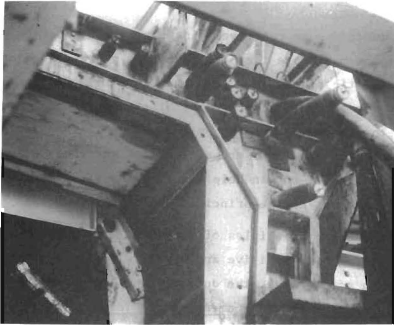
(a) Inflated duct stiffening and alignment tubes extending through far end of form
