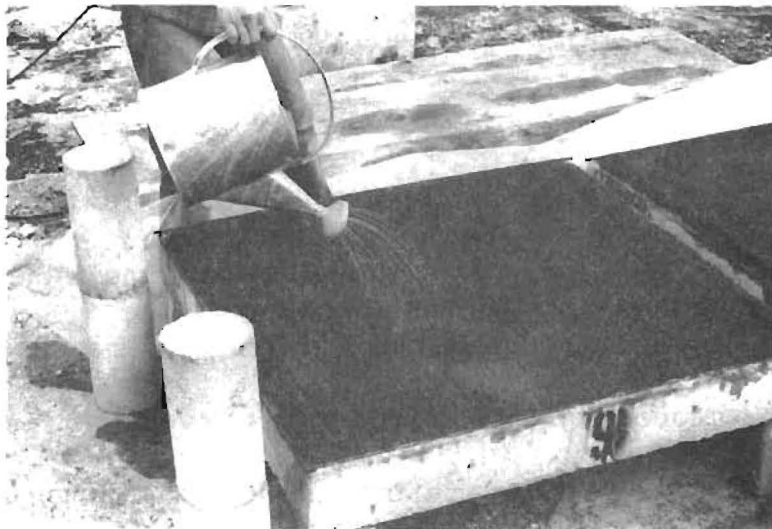
FIG. 3.2 APPLICATION OF MONOMER DURING FIELD TREATMENT OF SLOPED SLABS WITH FINE AGGREGATE COVER
