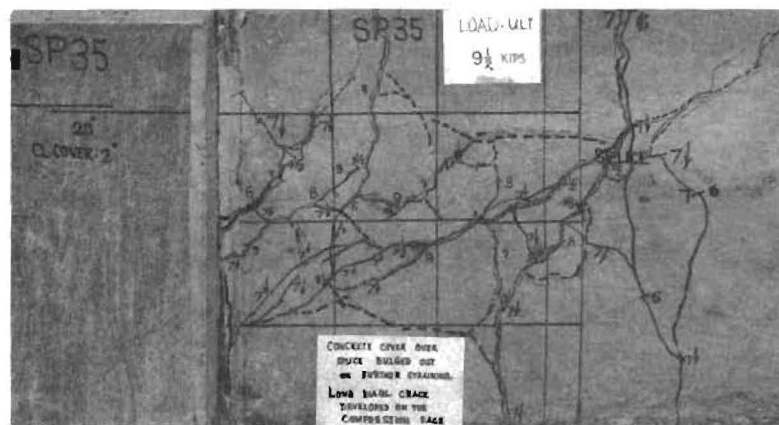
(b) Dashed lines mark cracks added at ultimate.
