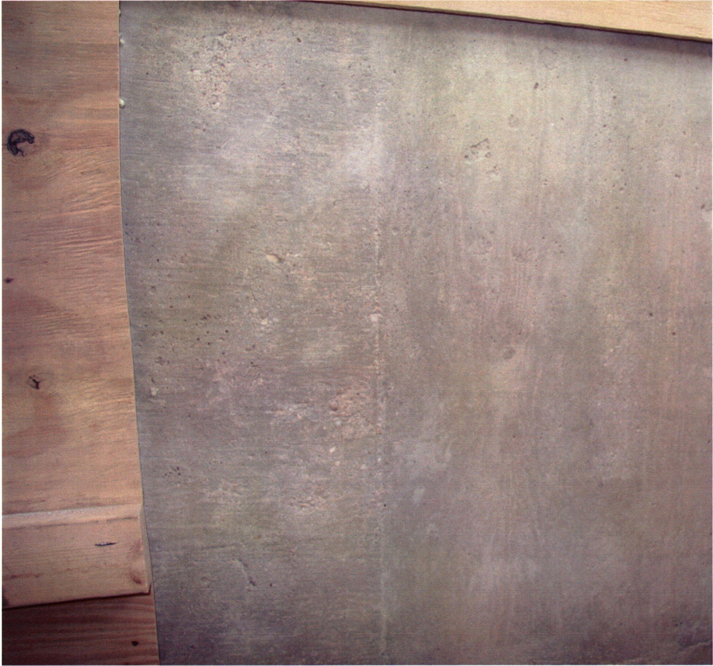
Areas cleaned by abrasive blasting. Some surface damage evident.
