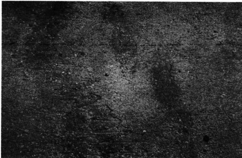
(b) Attempted to close cracks while Semi-plastic
